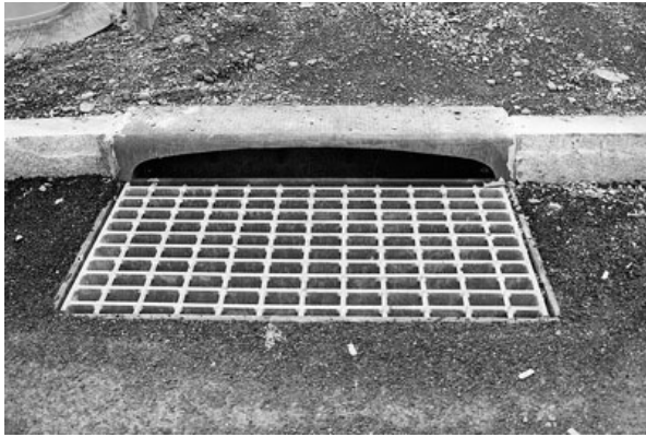
Figure 21. Bike Friendly Catch Basin Grate
