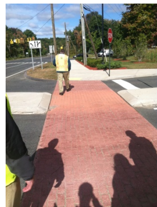
Figure 10. Mis-aligned sidewalk ramp
