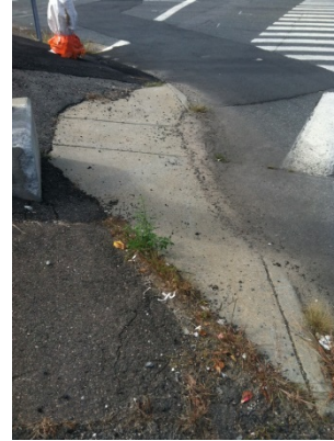
Figure 8. Steep sidewalk ramp
