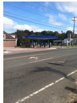
Figure 16. Faded pavement markings
