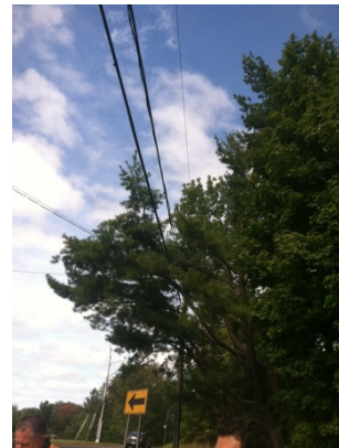
Figure 14. Tree branches around power lines
