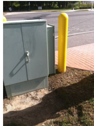
Figure 20 Telecommunications boxes adjacent to Dunkin Donuts sidewalk
