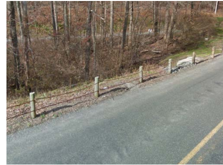
Figure 8. Cable guiderail system in need of upgrade.
