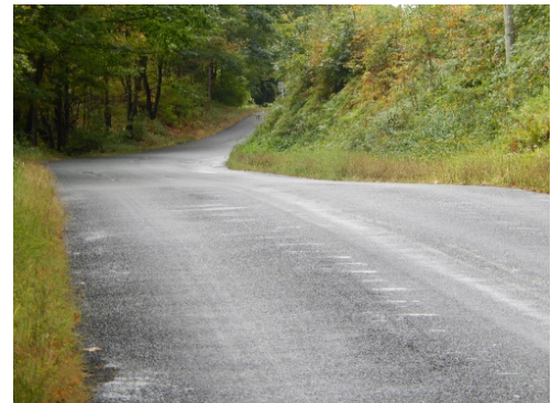
Figure 7. Ledges area / faded striping
