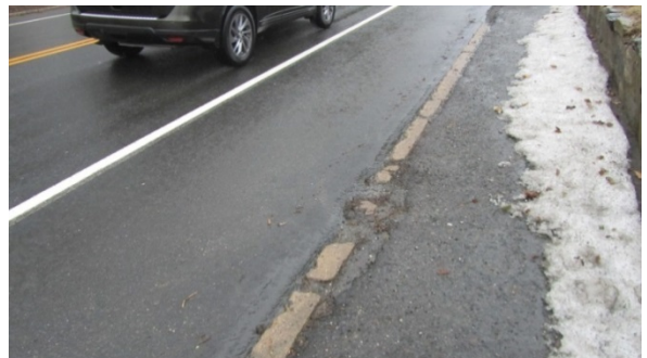
Figure 9: Snow and deteriorated curb on east side of Greenwood Road West northbound between curve and Station Place
