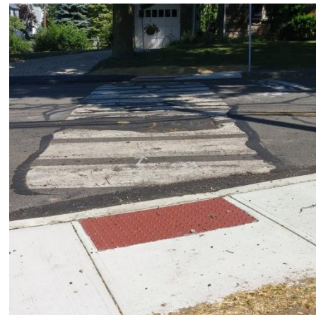
Figure 5. New Curb Ramps and Faded Crosswalk at Marvin St and Calf Pasture Beach Rd
