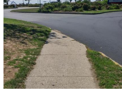
Figure 10. Curb Ramp Without Detectable Warning Strips
