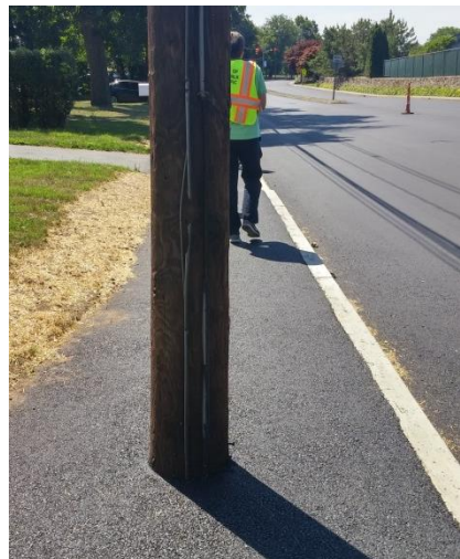
Figure 8. Repaved Sidewalk North of Elementary School With Utility Pole Obstruction
