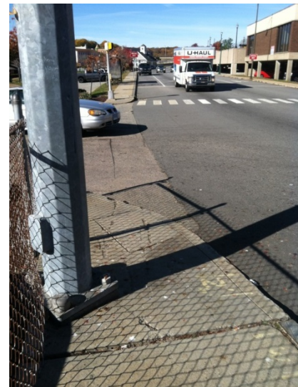
Figure 15. Mis-aligned handicap ramp
