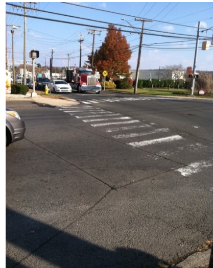
Figure 9. Faded crosswalks at intersection of Route 536 and Route 372
