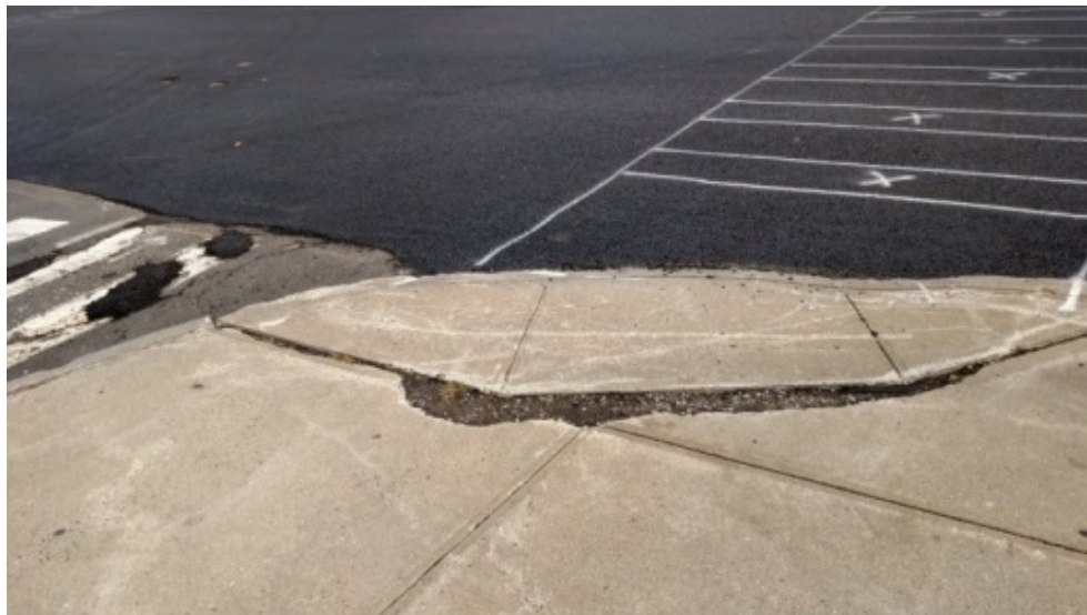
Figure 13 Ansonia RSA - Curb Ramp not ADA Compliant
