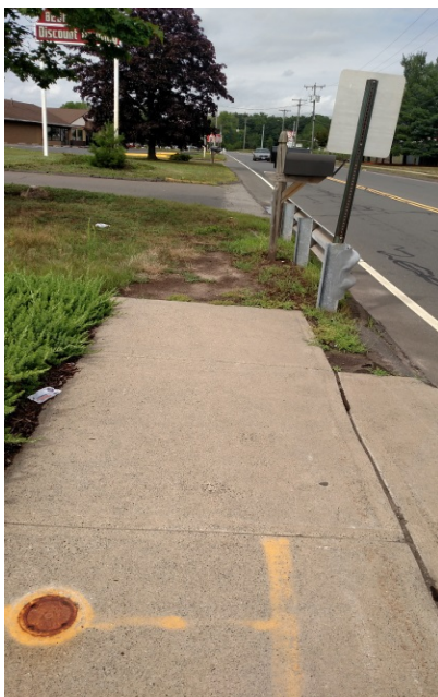
Figure 19 Southington RSA - Incomplete Sidewalk Network
