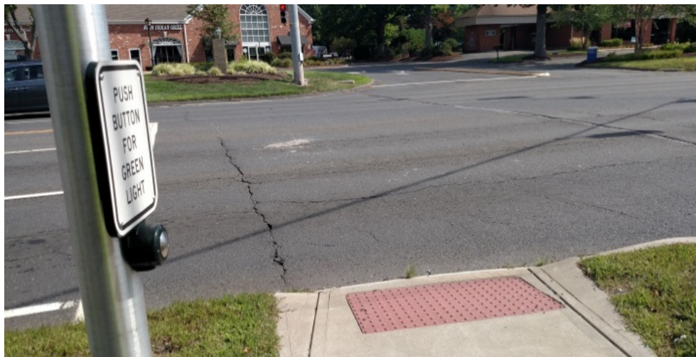
Figure 14 Avon RSA - Missing Crosswalk
