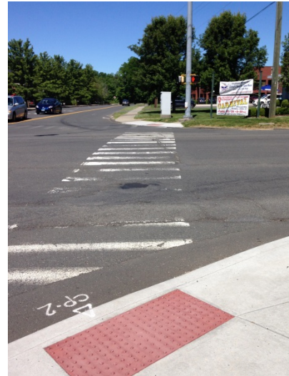
Figure 8. Existing ADA Ramps Not Compliant
