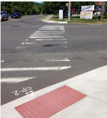
Figure 17. Realign Tactile Warning Strips to Face Direction of Crosswalk
