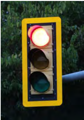
Figure 22. Signal with Retroreflective Backplate
