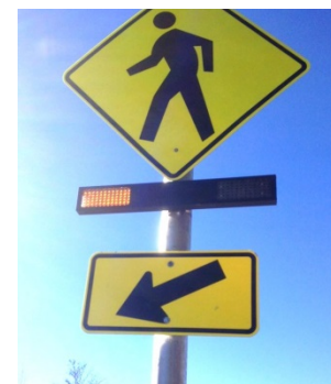
Figure 22 - Rectangular Rapid Flashing Beacon
