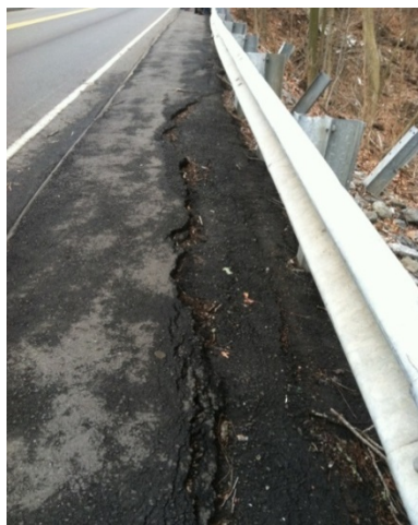
Figure 22: Washed out guiderail/degrading sidewalk
