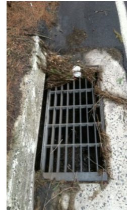
Figure 10: Non-bicycle friendly catch basin grate
