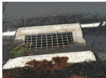
Figure 9: Clogged catch basin
