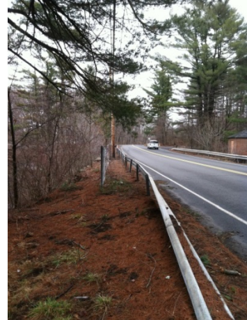
Figure 19: Narrow width between fence and guiderail
