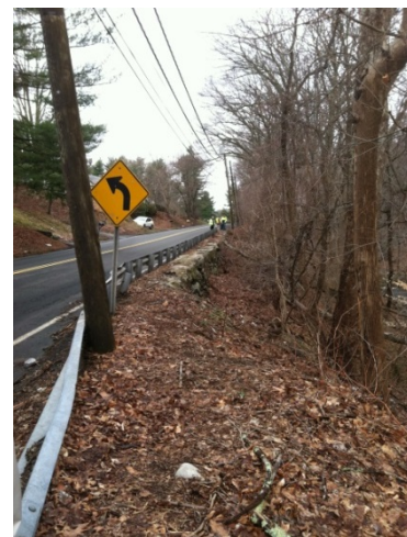
Figure 24: Sign behind utility pole
