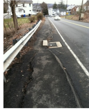
Figure 16: Catch basin encroaching into sidewalk
