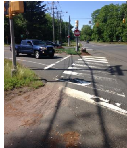
Figure 13. Triangular Channelizing island and Sand Buildup at Crosswalk.
