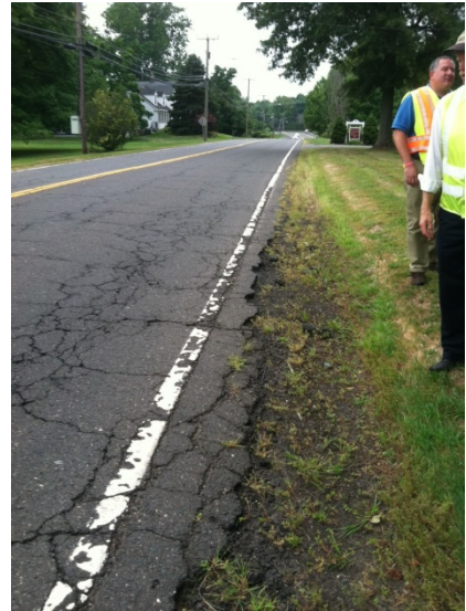
Figure 7. Broken Up Shoulder Pavement
