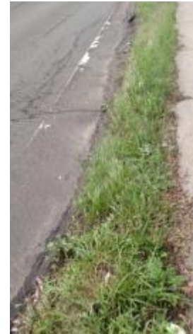
Figure 9. Missing Curb on Queen Street West Side Near I-84
