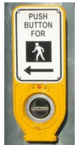
Figure 23. ADA Compliant Pedestrian Button
