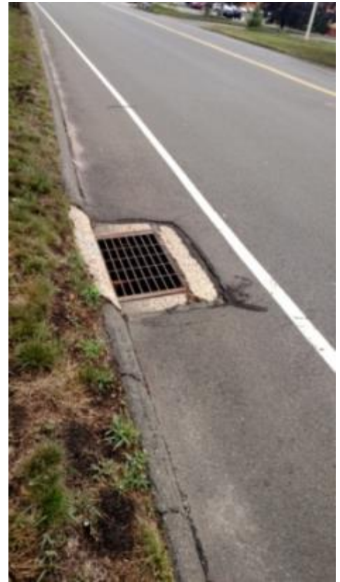
Figure 15. Non-Bicycle Friendly Catch Basin Grate.
