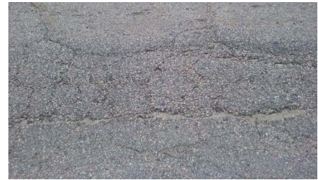
Figure 10. Pavement Cracking on Route 207
