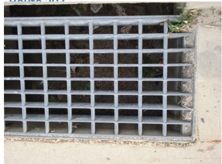
Figure 11. Catch Basin With High Sediment Levels
