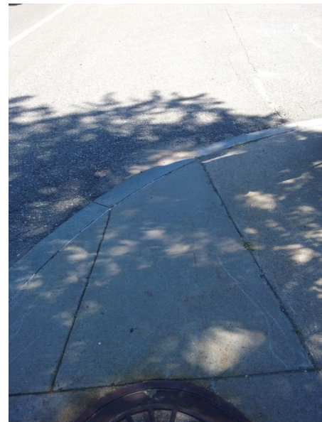
Figure 15. Sidewalk Ramp Which Does Not Meet Current Standards.
