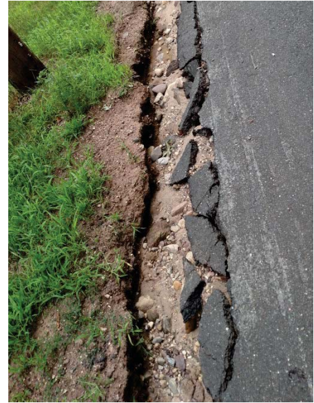
Figure 8. Rutting on Old Post Road
