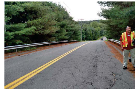
Figure 13. Poor Pavement Quality of Old Cathole Road
