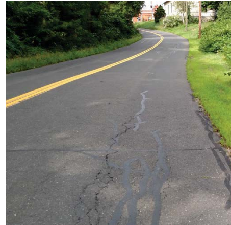
Figure 15. Deteriorating Condition of Old Post Road
