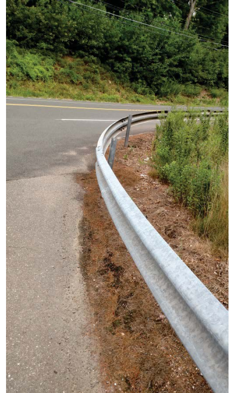
Figure 12. Loose Guard Rail
