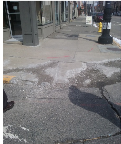
Figure 6. Broken Sidewalk Ramp
