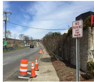
Figure 12. Vegetation Encroaching on the Sidewalk
