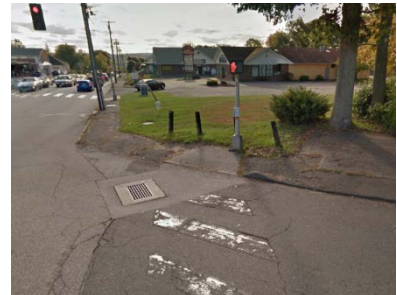
Figure 10. Non-Compliant ADA Ramp, Faded Crosswalk
