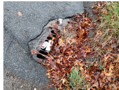
Figure 8. Clogged Catch Basin
