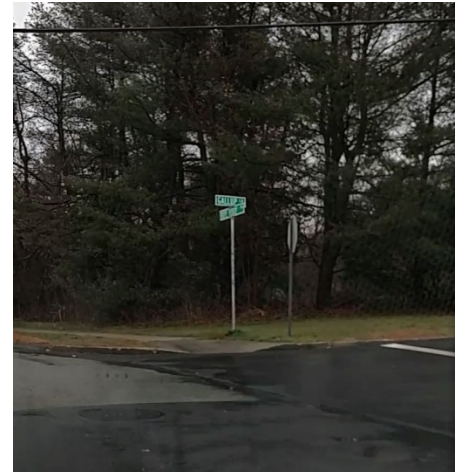
Figure 9. Lack of Tactile Warning Strip on Sidewalk Ramp
