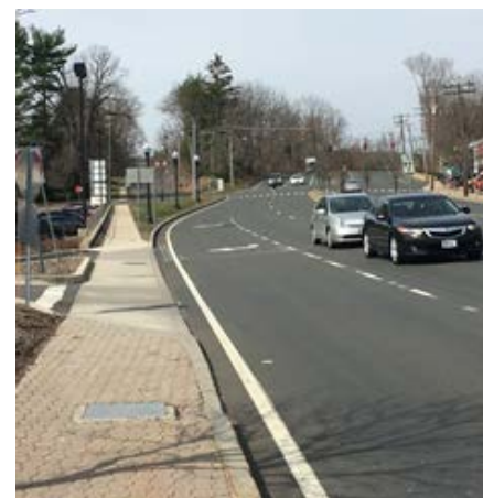
Figure 10. Inadequate Shoulder Area
