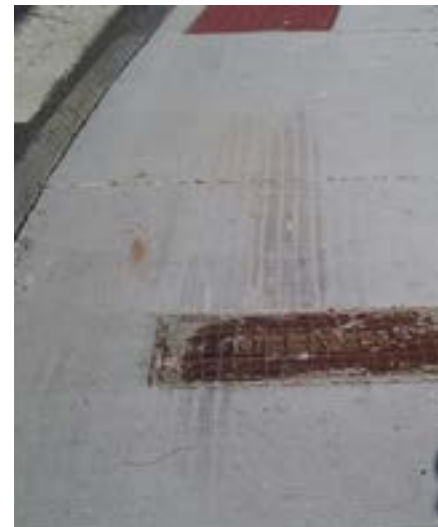
Figure 8. Tire Marks on Sidewalk
