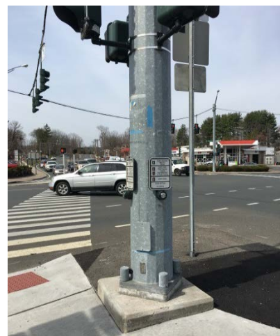
Figure 7. Unclear Pushbutton Direction
