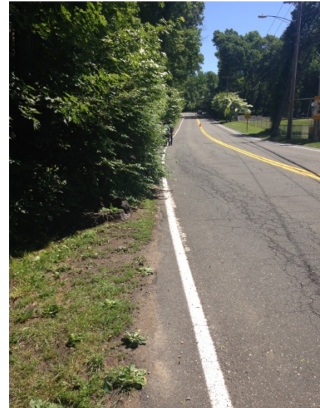
Figure 10. Overgrown Vegetation on School Road
