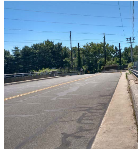
Figure 18. I-95 Bridge With Narrow Sidewalk and Wide Lanes
