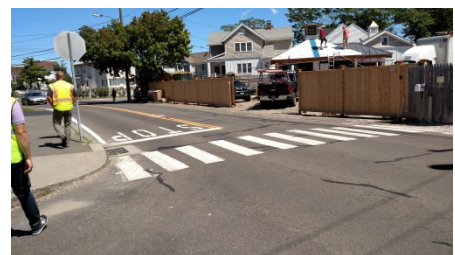
Figure 17. Crosswalk at Compo Hill Avenue Intersection Lacks Sidewalk Connection on the East Side
