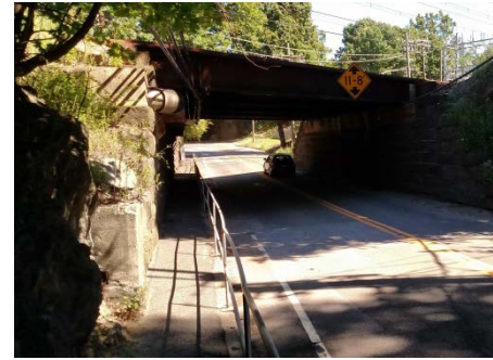
Figure 8. Narrow Sidewalk and Lack of Lighting Under the Metro North Bridge
