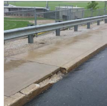
Figure 13. Broken Concrete Curb on North Side of Willow Street
