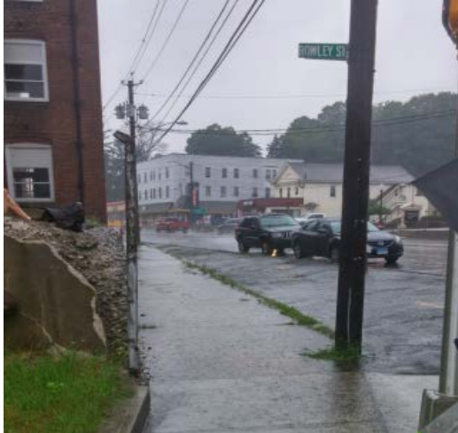
Figure 20. Water Running on sidewalk at Southwest Corner of Main Street/Rowley Street
