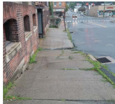
Figure 9. Poor Sidewalk Condition on Bridge looking North at Main Street
