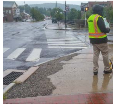
Figure 8. Deteriorating Sidewalk on Southwest Corner of Main Street/Bridge Street
