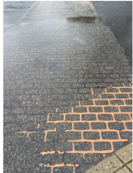
Figure 10. Worn Crosswalk Markings
