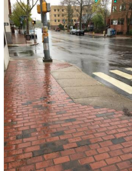
Figure 9. Missing Detectable Warning Strips
