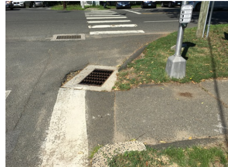
Figure 14. Crosswalks do not have a Ramp to Access Sidewalk
