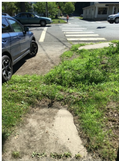
Figure 31. Complete Gaps in Sidewalks
