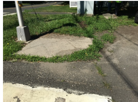
Figure 15. Ramp on Northeastern Side of Intersection is not Connected to Sidewalk
