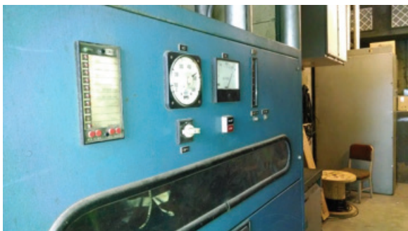
FIGURE 3-7: RECTIFIER (AT TIME OF THE PICTURE THE METERS READ 620V AND 475A)
