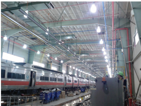
FIGURE 3-12: S&I SHOP INTERIOR LIGHTING
