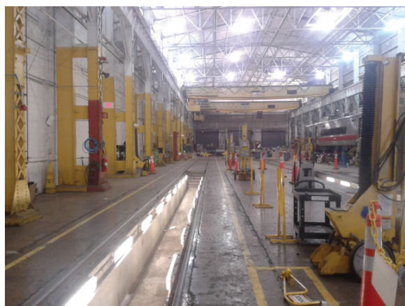
FIGURE 3-18: CSR SHOP WITH TWO 30-TON CRANES IN THE BACKGROUND MOUNTED ABOVE, AND ONE OF THE 25-TON JACKS TO THE RIGHT OF THE PHOTO
