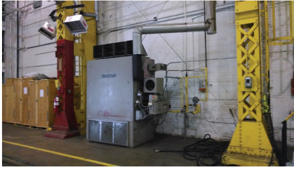
FIGURE 3-20: HASTINGS OIL-FIRED HEATER AND NATURAL GAS-FIRED HEATERS
