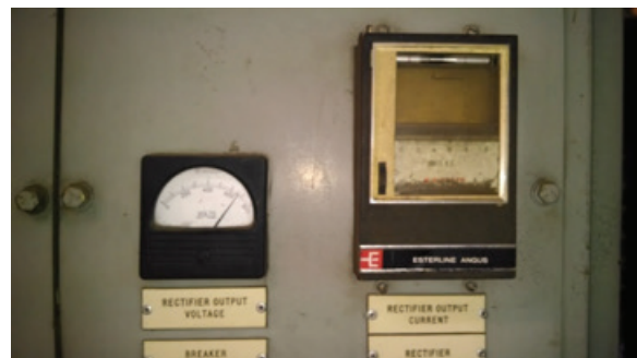
FIGURE 3-8: SECOND RECTIFIER (WHEN PHOTO WAS TAKEN 650V WAS DISPLAYED AND THE CURRENT METER WAS BROKEN)
