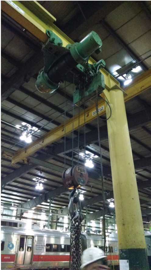
FIGURE 3-9: SEVEN AND A HALF TON CRANE
