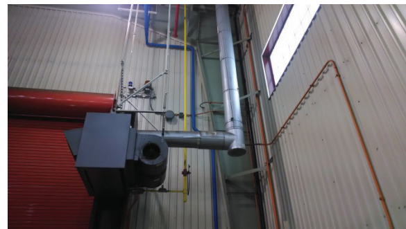
FIGURE 3-17: BLOWER BY BAY DOOR
