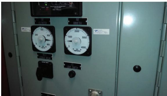
FIGURE 3-16: RECTIFIER (700V AT 570A)
