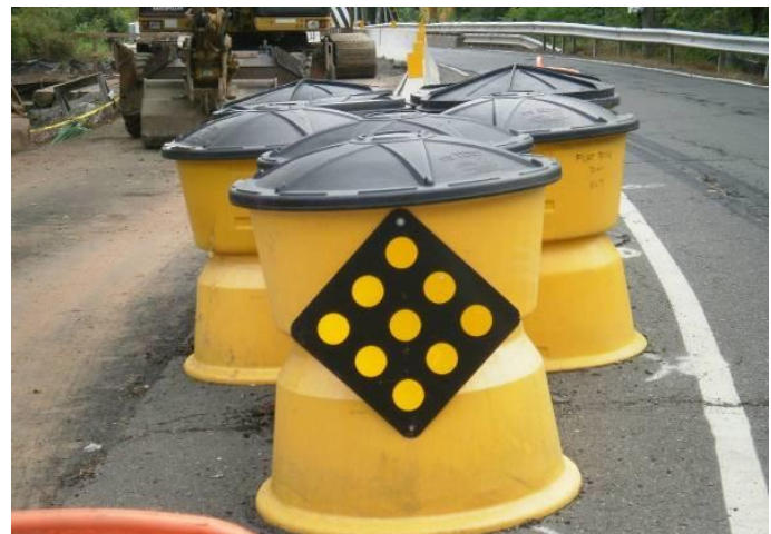
Temporary impact attenuation system protects blunt end of TPCBC.
