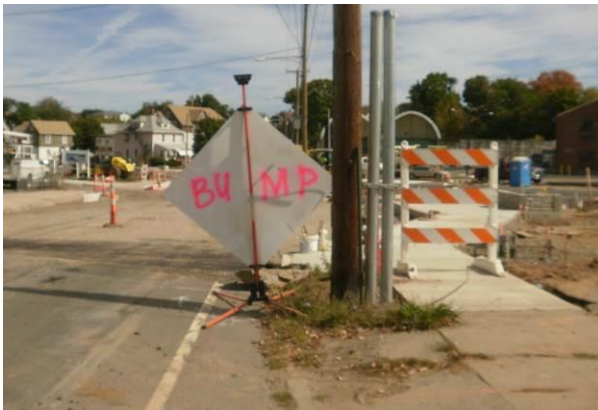
Two "Bump" signs were spray painted on the back of other signs due to theft of signs
