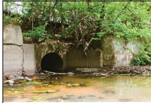
THE INTAKE OPENING ON THE NAUGATUCK RIVER FOR THE 1906 FACTORY WATER SUPPLY PIPE THAT RUNS BENEATH THE JACKSON STREET SITE.
