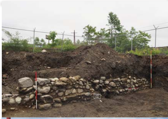
SOUTH FOUNDATION OF THE MACK HOUSE AT 25 JACKSON STREET. THE DISTURBANCE IN THE MIDDLE OF THE WALL IS WHERE A PORCH OR STOOP ONCE STOOD.
