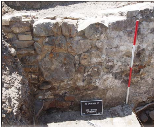
BASEMENT-LEVEL WINDOW OPENINGS AT 32 JACKSON STREET HAD BEEN FILLED IN WITH STONEMWORK AT SOME PERIOD, BUT THERE WAS EVIDENCE OF PLASTERING ON THE INTERIOR BRICK AND STONE FOUNDATION WALLS.
