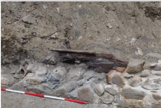
FOUNDATION AT 23 1/2 JACKSON, SHOWING THE LOCATION OF A WINDOW WELL WITH A DISPLACED WOODEN SILL, AND TO THE LEFT A SANITARY PIPE EXTENDING THROUGH THE FOUNDATION.
