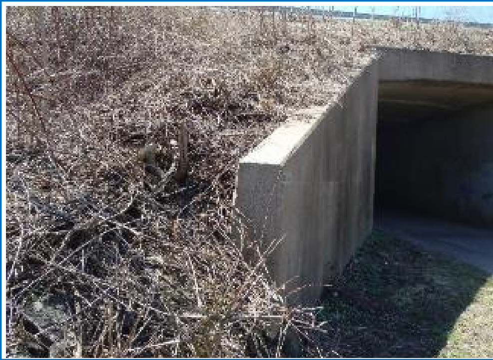
Southeast Wingwall (Note: Area of erosion behind)
