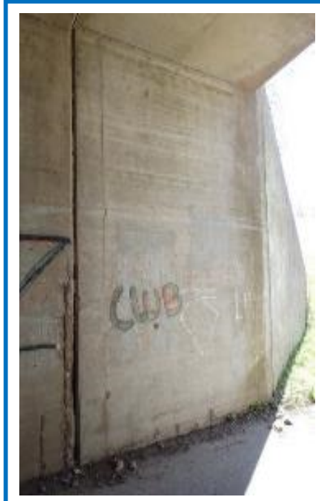
Panel 1 Southwall (Note: Spall with exposed reinforcement)
