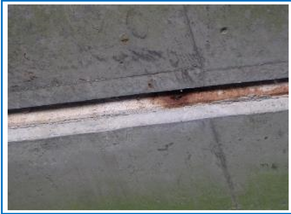
Vertical Misalignment between Panels 10 & 11 up to 3”
