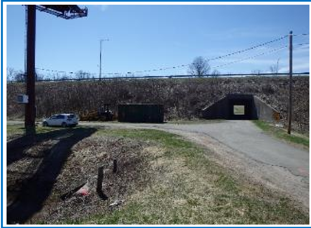
East Roadway Leading up to Bridge (Note: Drainage structure and aerial electrical feed for billboard)
