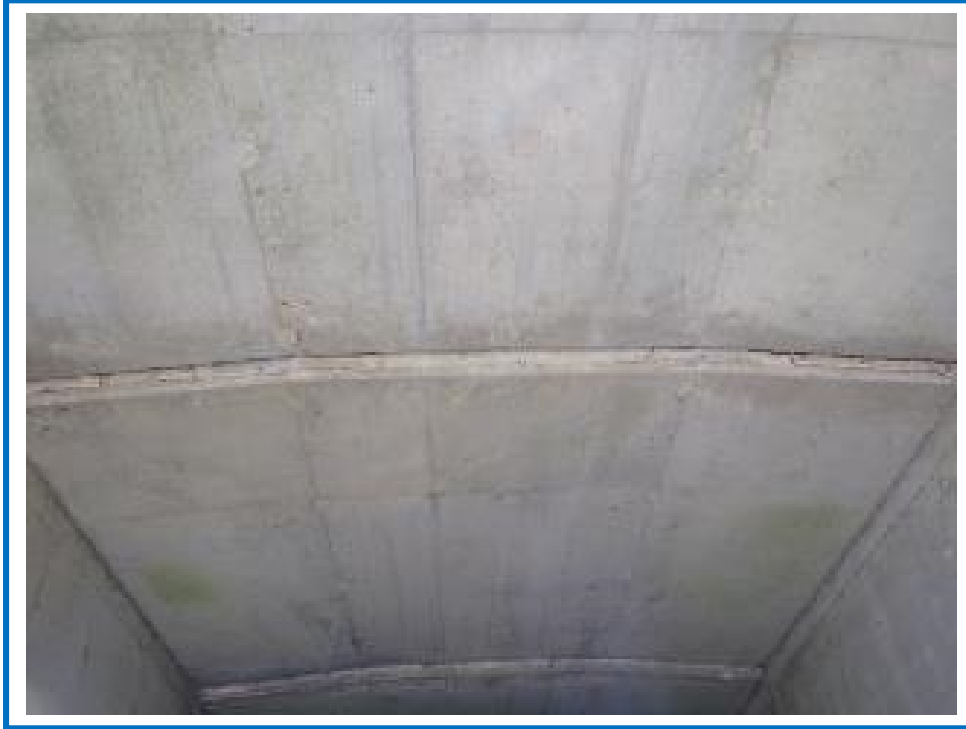
Joint at Roof Panels 1 & 2 (Note: Misalignment typical in first and last four spans)
