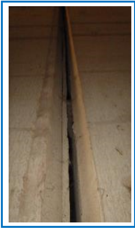
Typical Vertical Joint with Gap (Note: Joint between panels 6 and 7 south wall shown)
