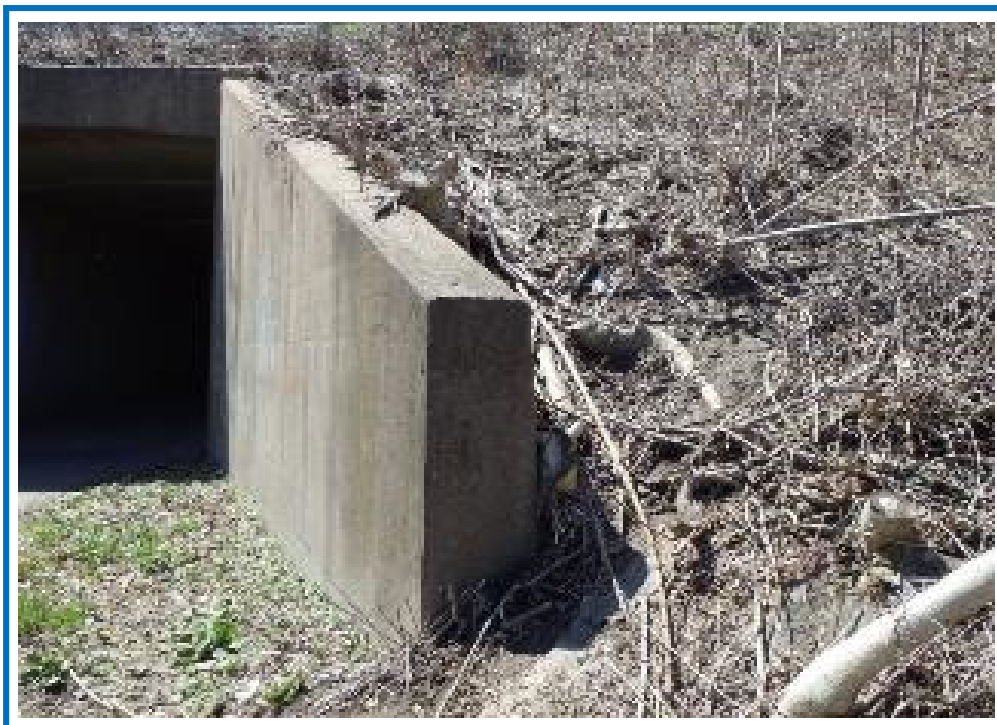
Northeast Wingwall (Note: Area of erosion behind)
