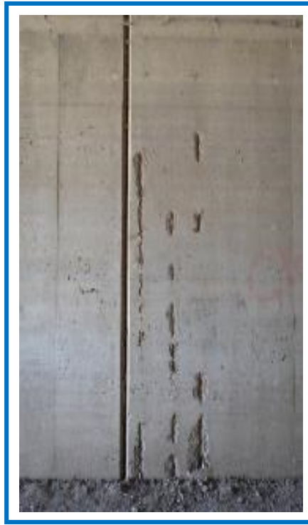
Panel 8 at Joint 8 South Wall (Note: Spalls and gap in joint)
