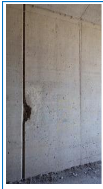
Panel 9 North Wall at Joint 8 with Spall and Exposed Reinforcement
