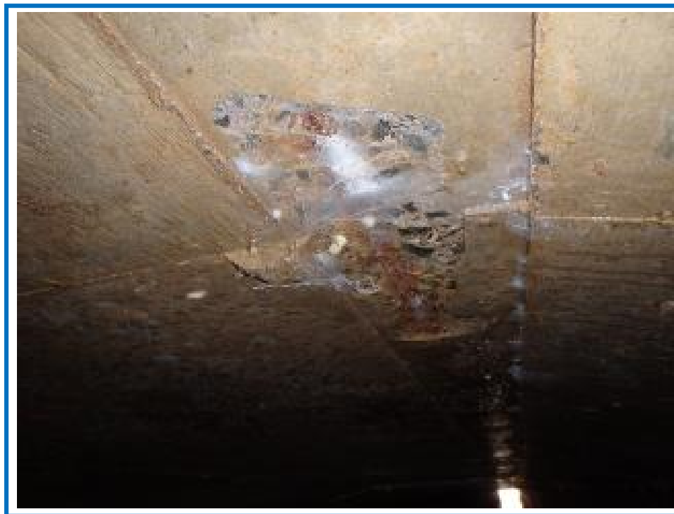
Spall at Top Panel 10 (Note: Exposed rusted reinforcement)
