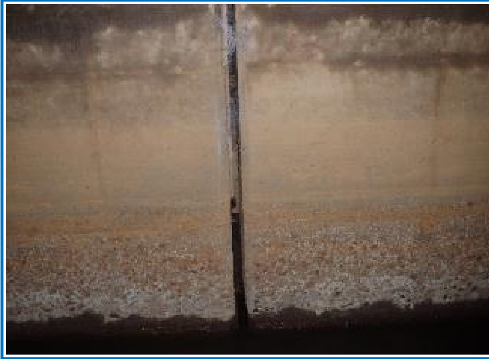
Joint 5 at South Panel (Note: Up to 2.5" wide gap between panels)
