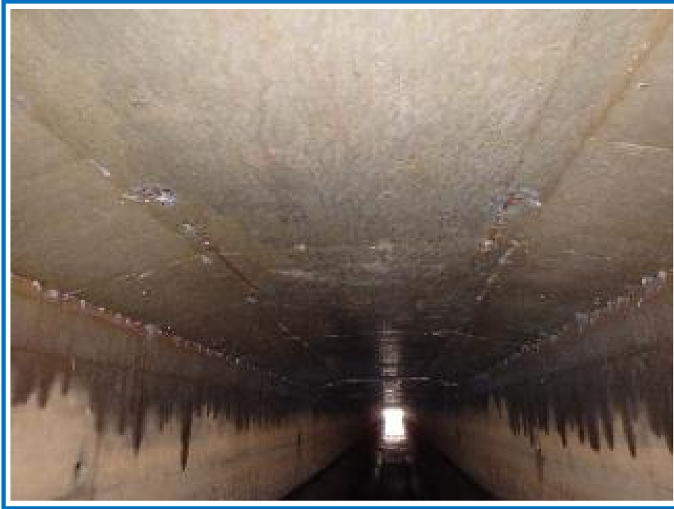
Top Panel 10 (Note: Spalls with exposed rusted reinforcement)
