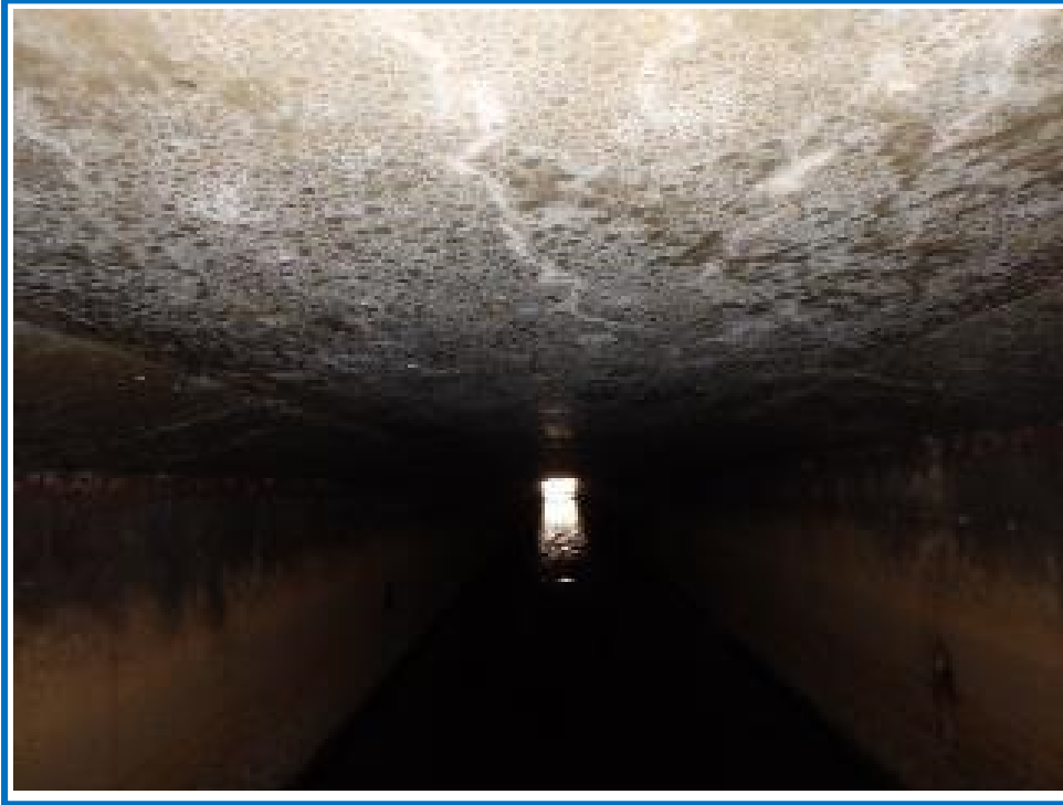
Top Panel 8 (Note: Scaling and heavy efflorescence)
