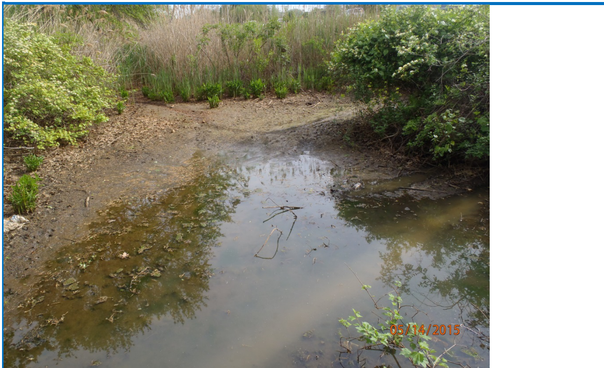
10: Headwall looking upstream Note vegetation blocking channel
