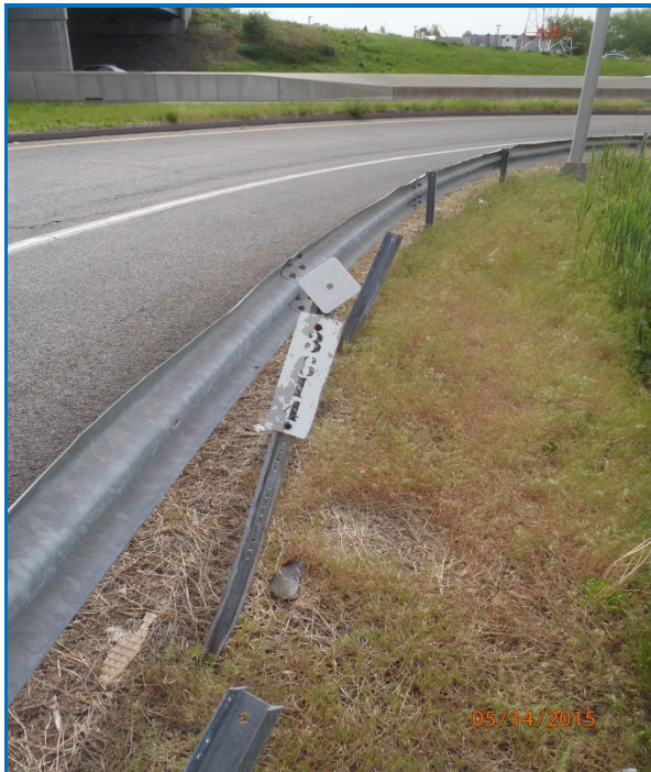
6: TR-828, Damaged MBR at right EOR
