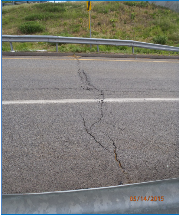
5: TR-828, Transverse cracks in bituminous
