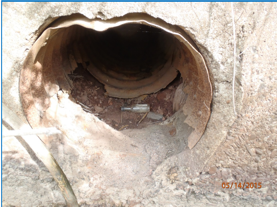
8: CMP at Southwest Wingwall Note section loss of pipe
