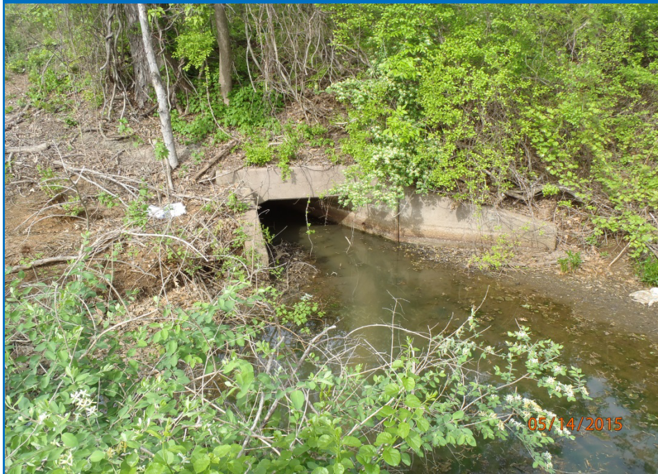
2: North Headwall, Inlet Note erosion at both wingwalls
