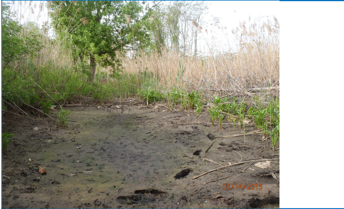
9-: Outlet looking downstream Note vegetation blocking channel
