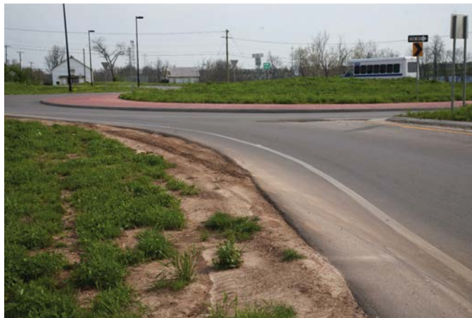
Exhibit 9.25. Evidence of vehicle encroachment on exit.
