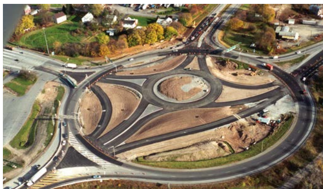
LOCATION: Albany Avenue/Broadway/I-587, Kingston, New York. SOURCE: New York State Department of Transportation, as shown in NCHRP Report 672 (1) .
