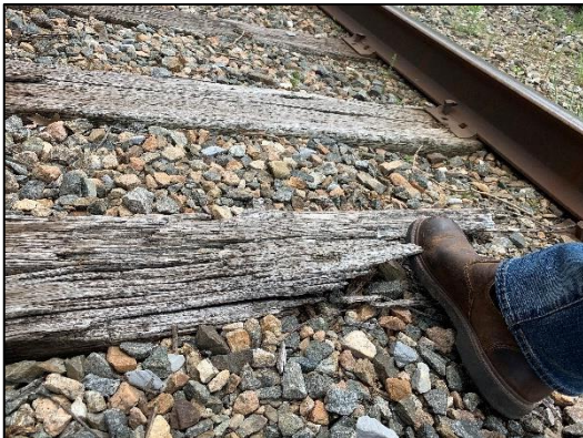
Figure 3: Severe Rotting of Wooden Ties - Lower Bartlett Road (MP 5.05)
