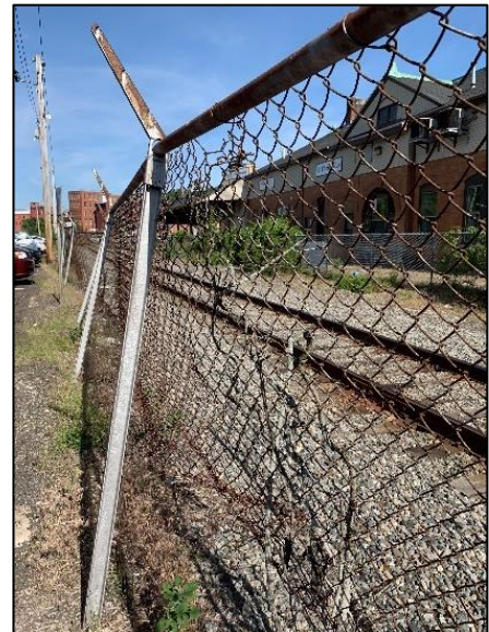
Figure 45: Damaged Fencing at Old Norwich Train Station (MP 12.3)
