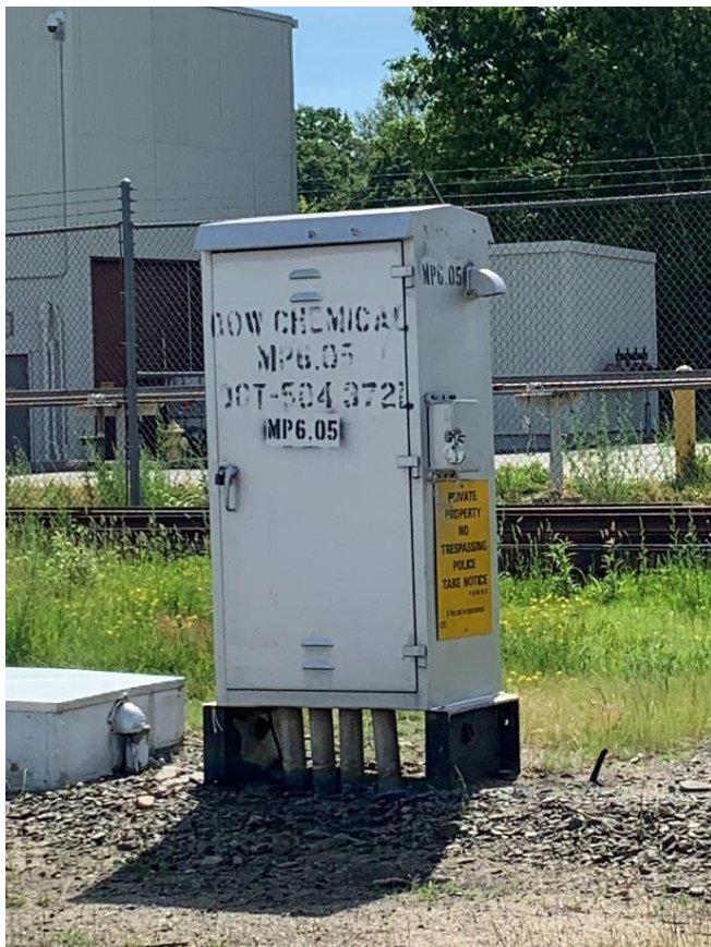
Figure 112: MP 6.08 - Grade Crossing - DOW Chemical (Cabinet)
