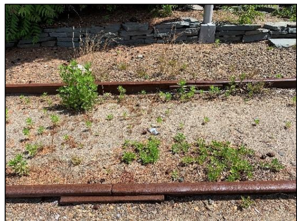
Figure 13: Lack of Visible Ballast/Ties and Vegetation Growth
