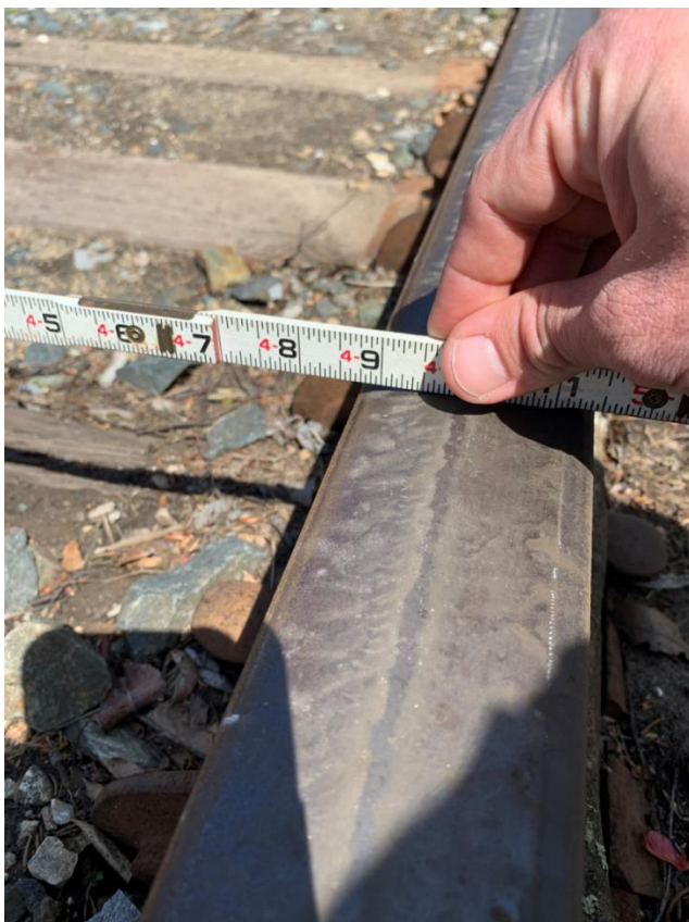
Figure 38: MP 2.37 – Track - Bentham Avenue – Measure of Track Gauge
