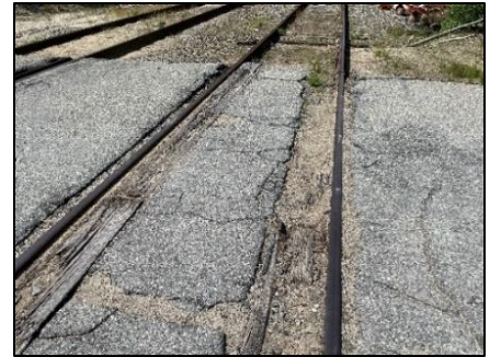
Figure 32: Fair Condition - DOW Chemical (MP 6.08)
