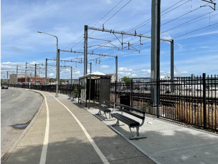
Figure 4: MP 122.90 – Power – New London Station - Shore Line is Equipped with Overhead Contact System
