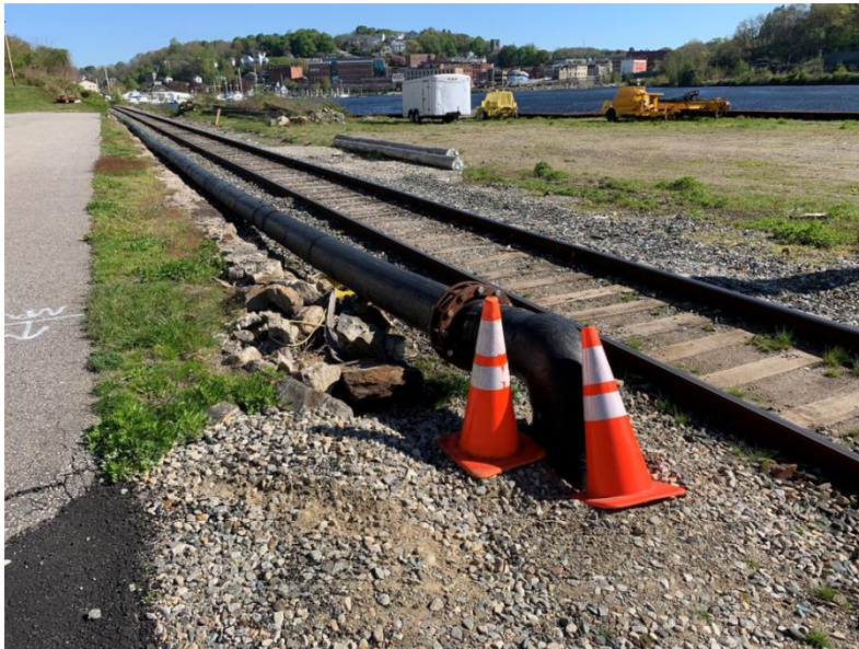
Figure 88: MP 13.00 – Utility - S Thames Street - Exposed Pipe running Alongside the Tracks (Looking North)
