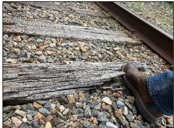
Figure 12: Wooden Ties with Severe Rotting
