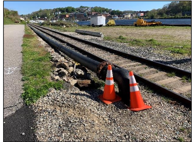
Figure 46: Exposed Outlet Sewage Pipe (Norwich)
