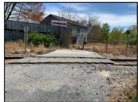
Figure 7: Grade Crossing with Severe Heaving (MP 5.05)
