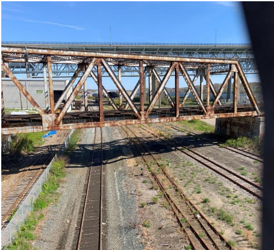
Figure 14: MP 0.62 – OH Bridge - State Pier Road (Looking North) - Amtrak Bridge and Two I-95 Bridges
