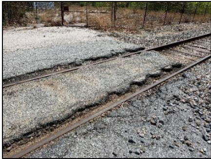
Figure 34: Poor Condition - Lower Bartlett Road (MP 5.05)
