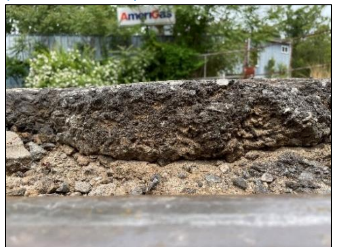
Figure 30: Elevation of Heaving from Rail Surface (Lower Bartlett Road)
