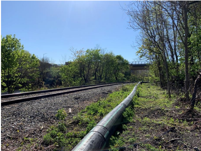
Figure 94: MP 13.50 – Track - North Thames Street (Looking North) - Exposed Piping
