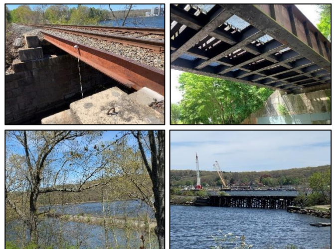
Figure 8. I-Beam Bridge (Top Left), Open Deck Bridge (Top Right), Thru Girder (Bottom Left), Timber Trestle (Bottom Right)
