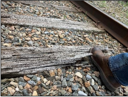
Figure 7. Wooden Ties with Severe Rotting
