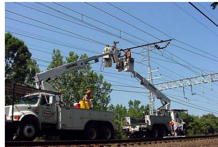
Figure II-2. NHL Catenary Line
