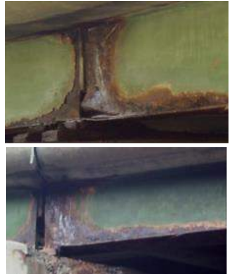
Figure 1. Typical End Corrosion of Bridge Girders [Photos Courtesy of Michael P. Culmo]
