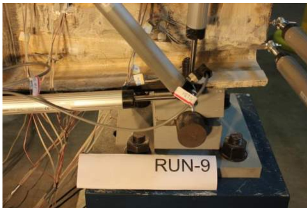
Figure B.2.42 Damaged Girder Bearing: +0.75 in
