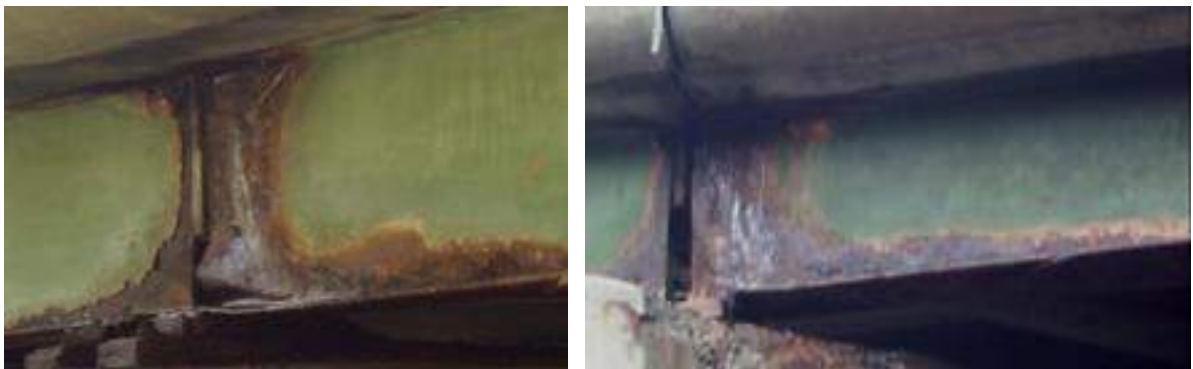
Figure 1.2 Typical End Corrosion in Steel Girder Ends (Photos: Michael P. Culmo)
