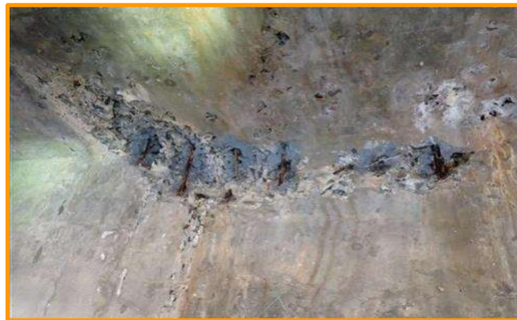
Spalls with exposed stirrup (Beam 5)
