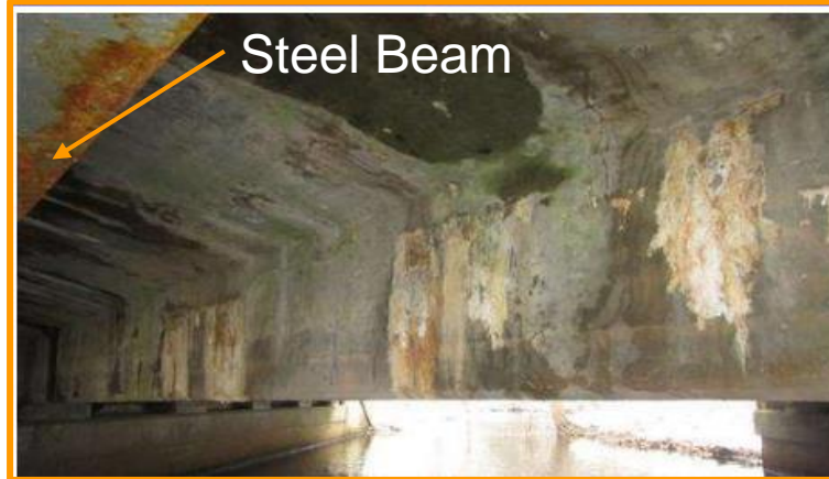
Active leakage at deck joint & efflorescence
