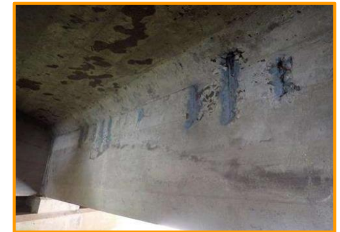
Spalls with exposed stirrups (Beam 5)
