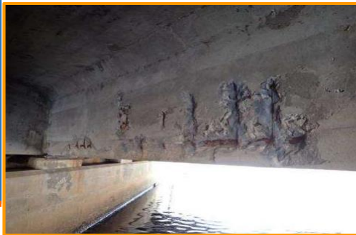
Spalls with exposed stirrup (Beam 3)
