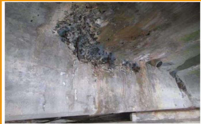
Spalls with exposed stirrup & honeycombing
