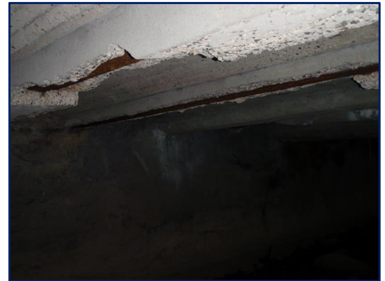
DETERIORATED CONCRETE ENCASED BEAM
