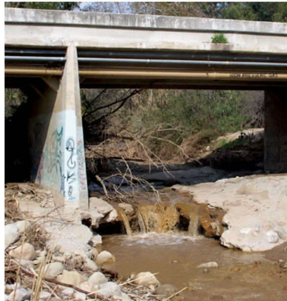
Scour occurring in the stream bed around a bridge pier
