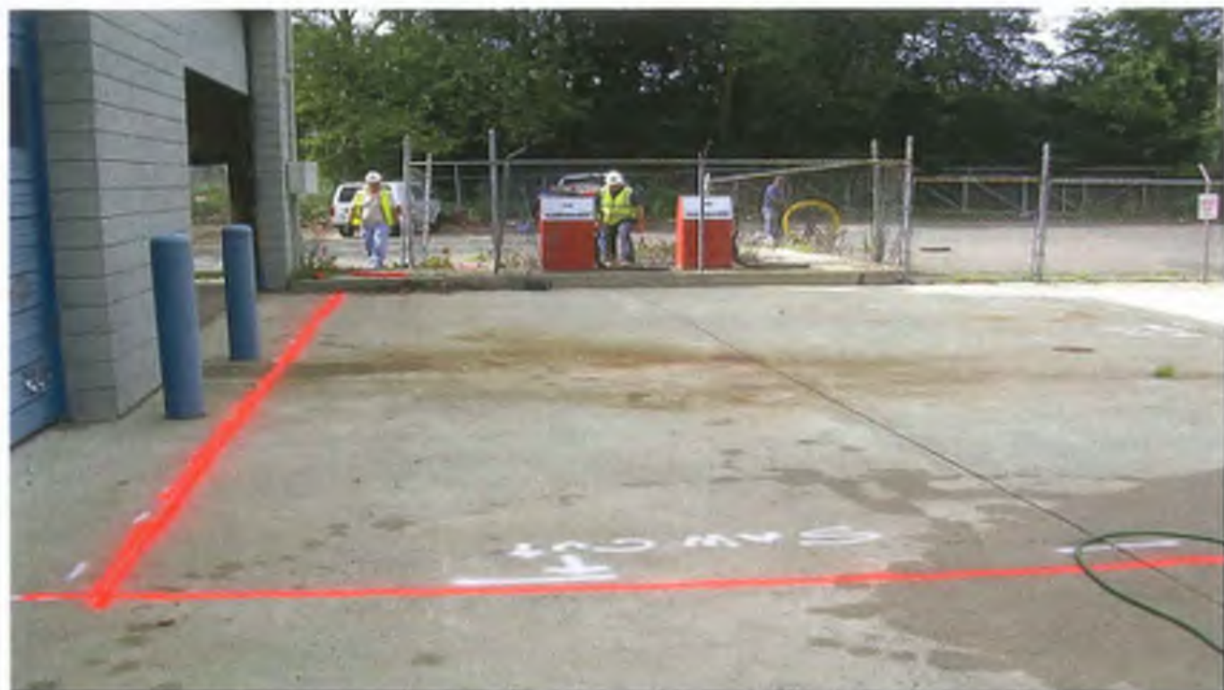
Photo 1: Removal of former fuel dispensers and security fence enclosure, proposed excavation outline for the removal of UST #1 and #2.
