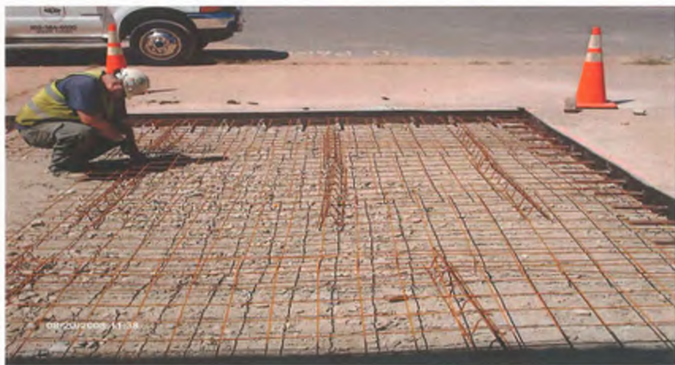
Photo 20: Installation of rebar dowels along edge of existing concrete pad, and welded wire fabric with step supports for replacement concrete pad (former USTs #1 and #2 area).
