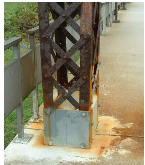
Catenary Repaired But Still Rusty
