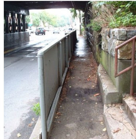
Narrow Walk under Railroad Bridge with Plywood Barrier
