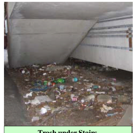
Trash under Stairs
