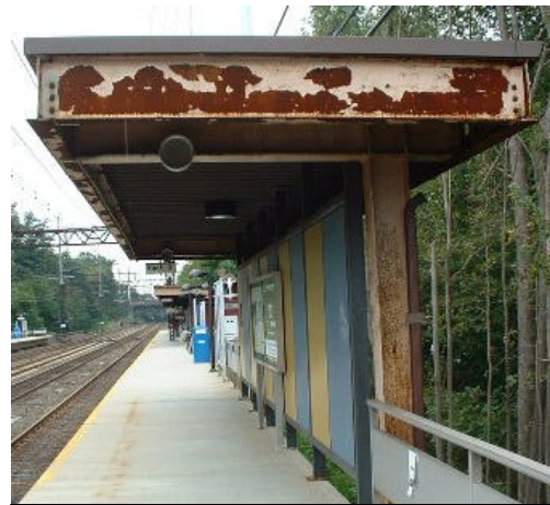
Canopy in Need of Paint
