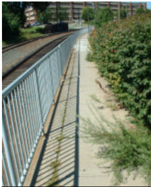
Walk & Railing with Overgrown Vegetation
