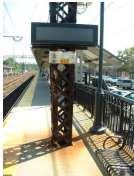
Catenary Support in Platform
