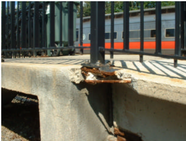
Concrete Spall and Poor Connection
