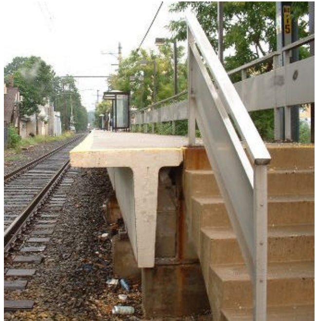
Glenbrook - Gap between Platform Edge and Stair Handrail
