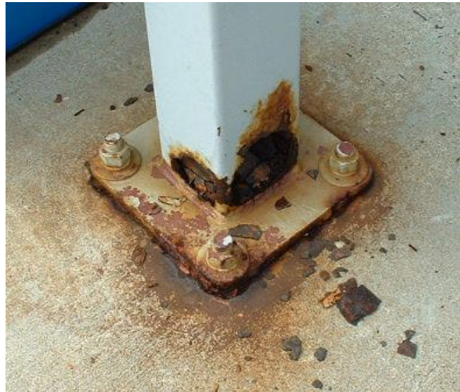
Rust Light Pole Base
