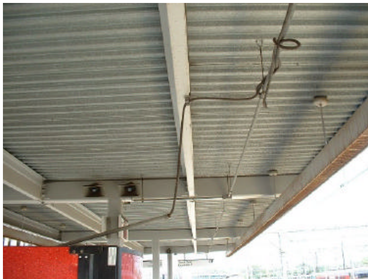
Power Feed Hanging from Canopy
