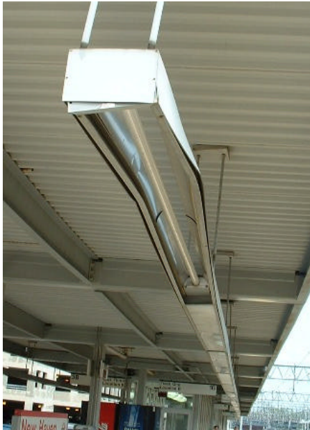
Broken Canopy Lights
