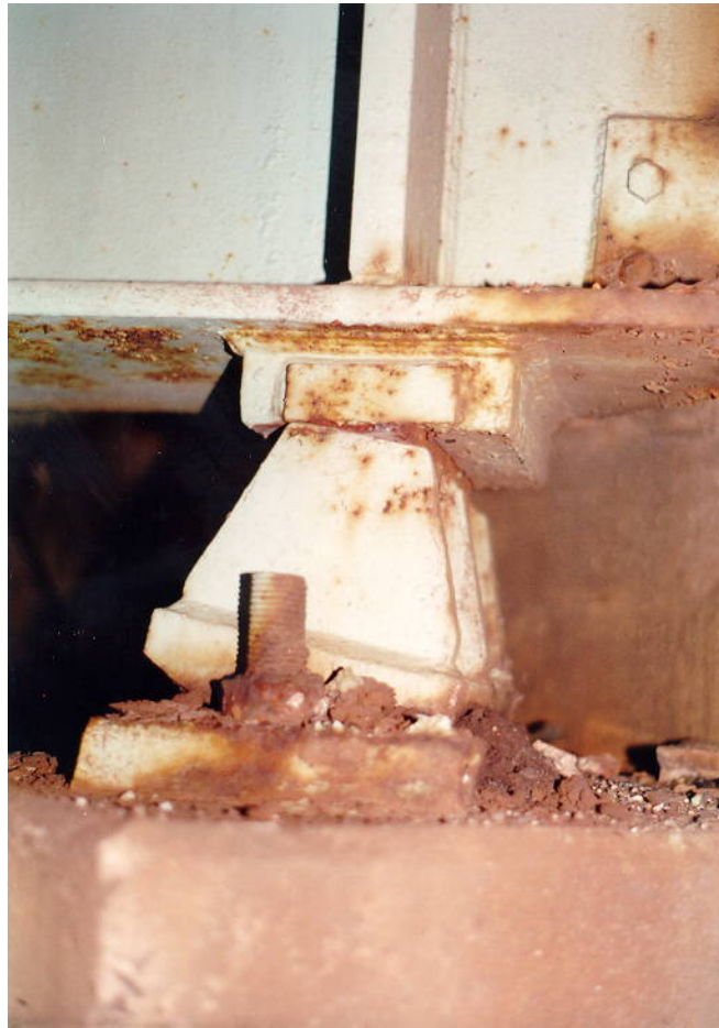
Figure 6.2.1i – Over Extended Rocker Bearing.
