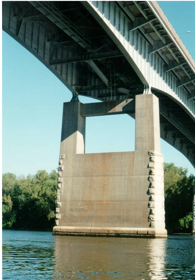
Figure 6.3.1b – Tall Concrete Pier with Decorative Stone Masonry Facing.
