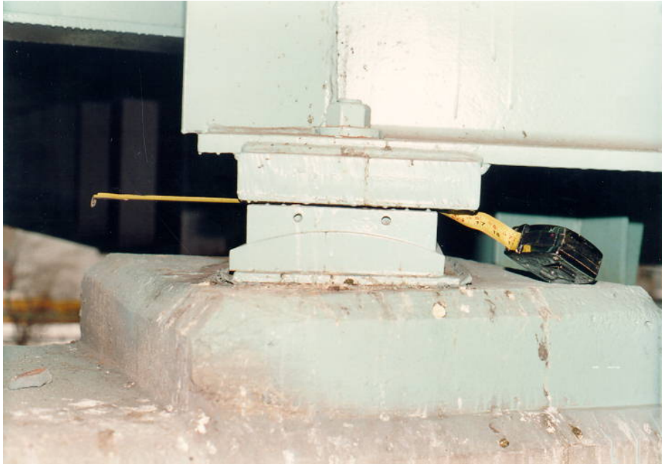
Figure 6.2.1j – Bronze Sliding Plate Bearing with a Gap Between the Sole Plate and the Sliding Plate.
