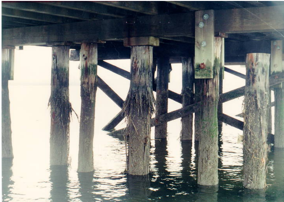
Figure 6.3.3a – Timber Pile Bent with Freeze-Thaw Damage in the Tidal Zone.
