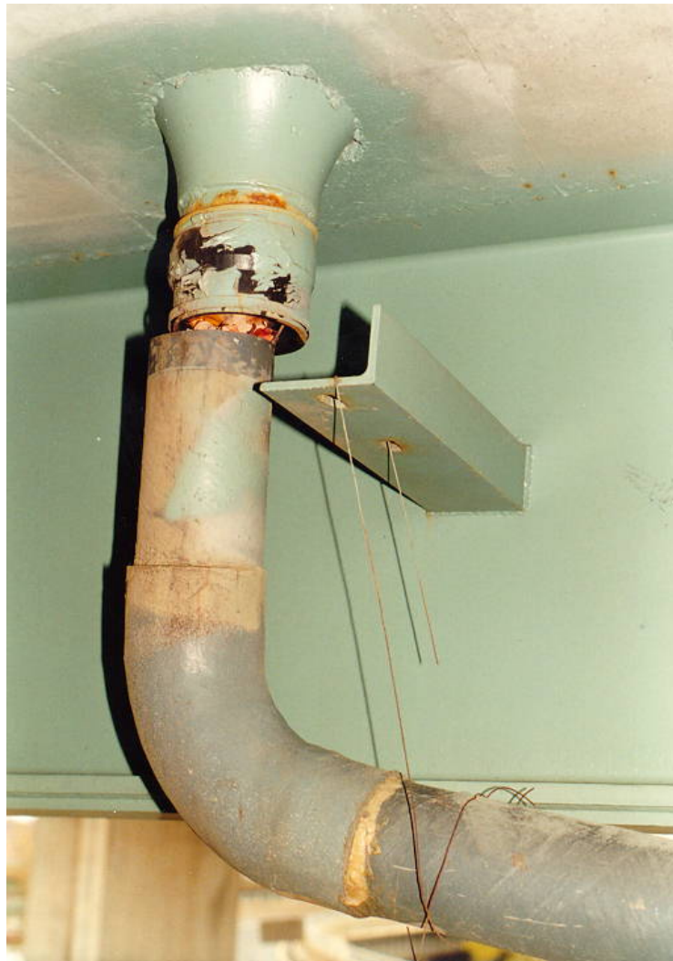
Figure 6.1.10a – Downspout Pipe Disconnected at Scupper Connection.
