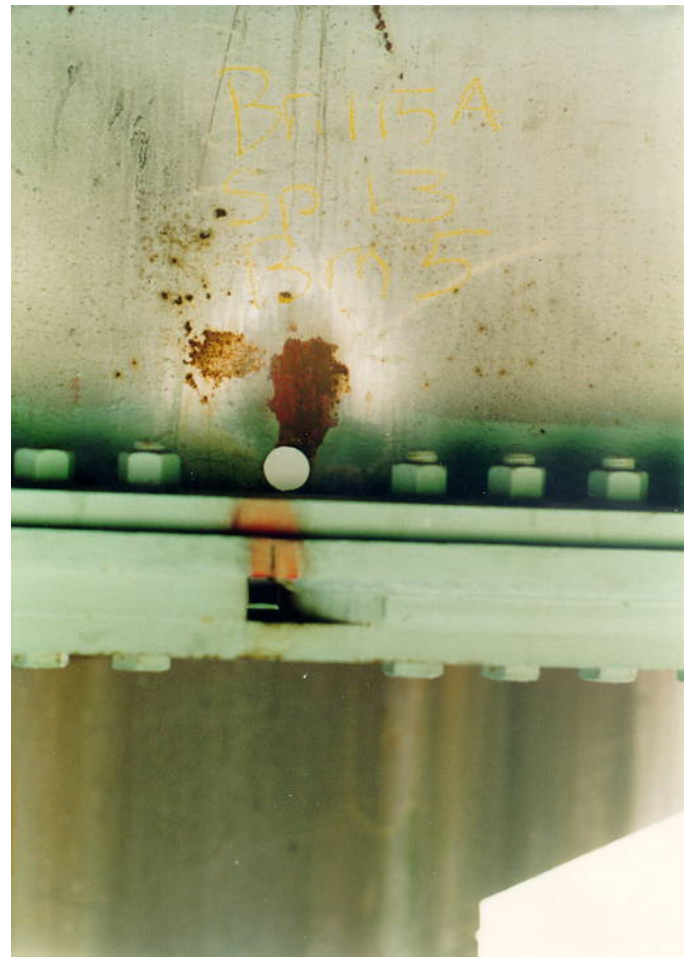
Figure 6.2.7.1c – Fatigue Crack Through the Bottom Flange of a Rolled Stringer at the End of a Partial Length Welded Cover Plate. A Stop Hole Has Been Drilled in the Web and Splice Plates Have Been Bolted to the Bottom Flange
