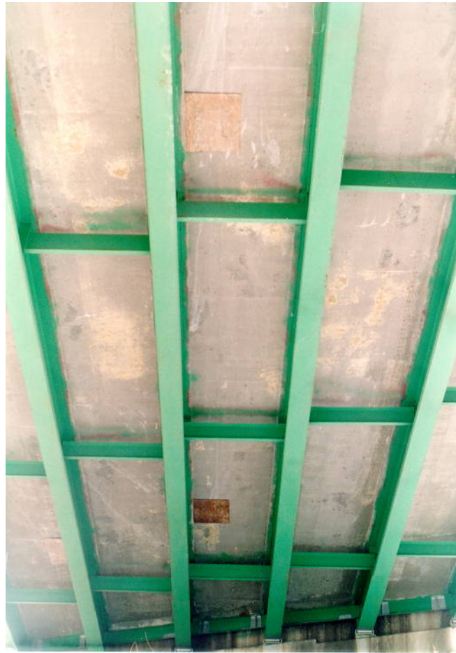
Figure 6.1.2c - Typical Underside of Concrete Deck. Note Cracking with Efflorescence and Formwork Remaining from Full Depth Patching.
