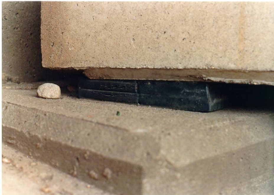
Figure 6.2.1m – Elastomeric Bearing. Note the Uneven Bearing Surfaces Causing Bulging and Cracking at the Rear of the Elastomeric Bearing Pad.
