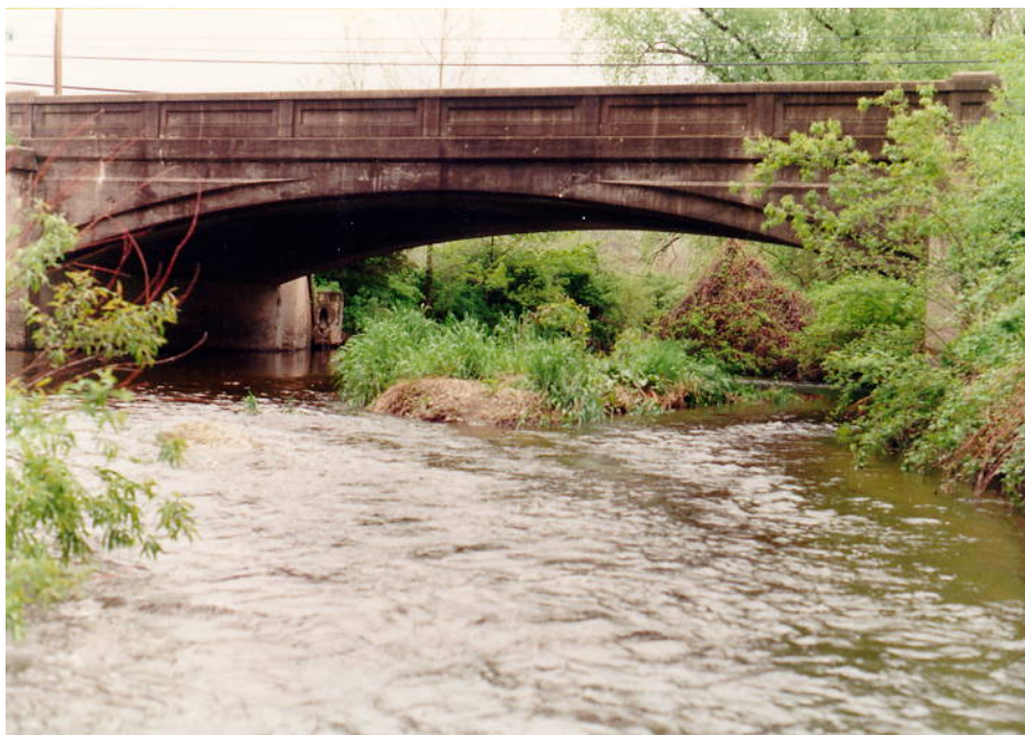
Figure 6.4.1b – Sand Bar and Vegetation Growth in the Channel.
