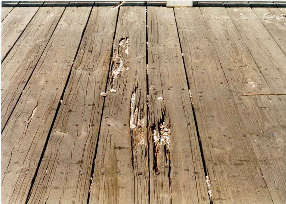
Figure 6.1.1a – Deterioration of Timber Plank Deck Surface
