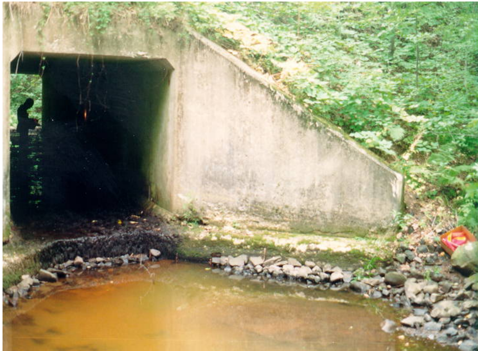
Figure 6.5a - Cast-In-Place Concrete Culvert with Erosion at the Outlet.
