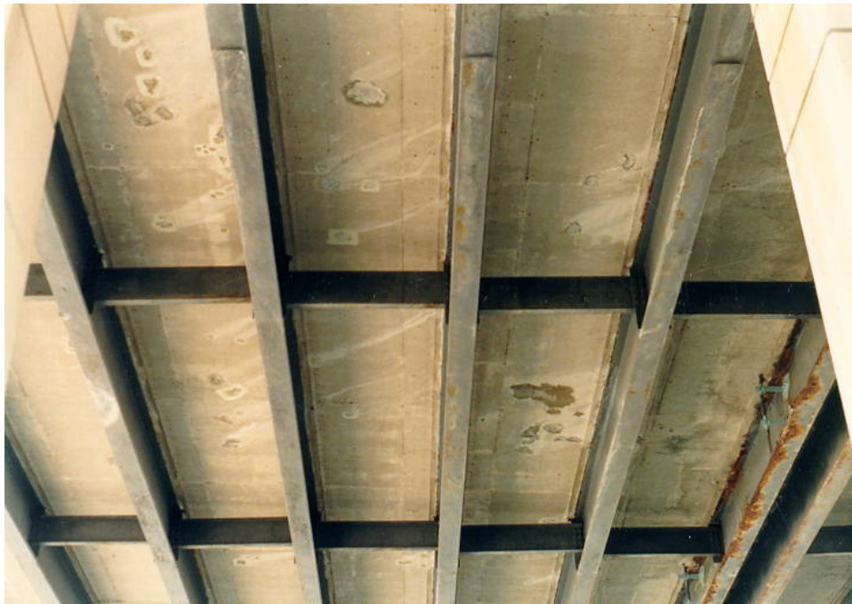
Figure 6.2.7a – Typical Rolled Multi-Stringer Superstructure with Ends of Partial Length Welded Cover Plates Visible.
