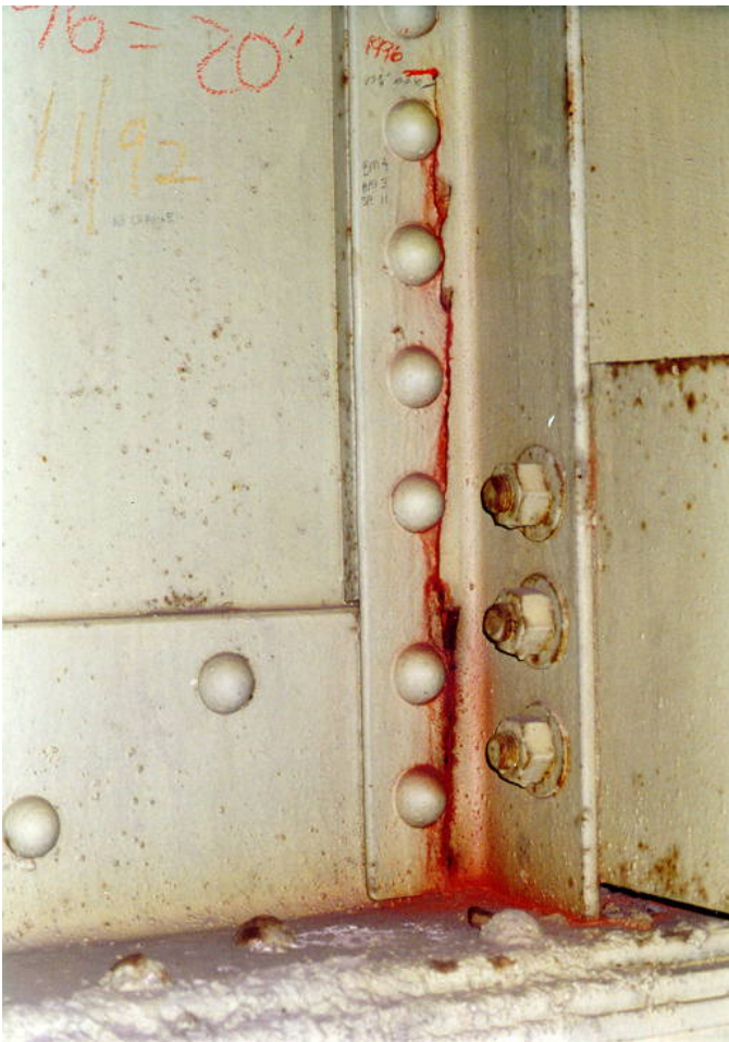
Figure 6.2.7.1b – Fatigue Crack in a Diaphragm Connection Angle on a Girder.
