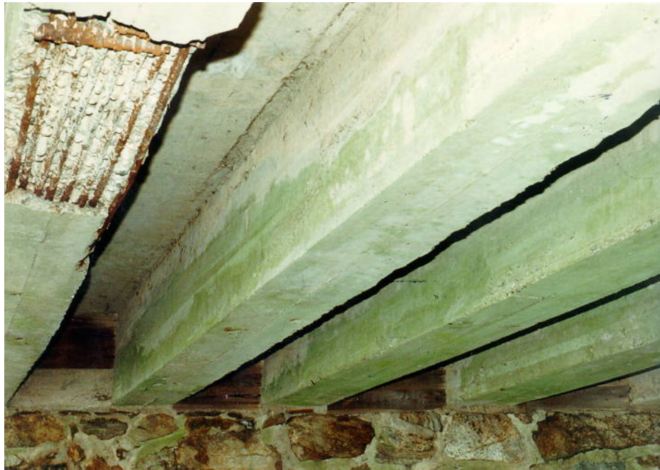
Figure 6.23a – Concrete T-Beams with Large Spalls Exposing the Bottom Layer of Reinforcing Steel.
