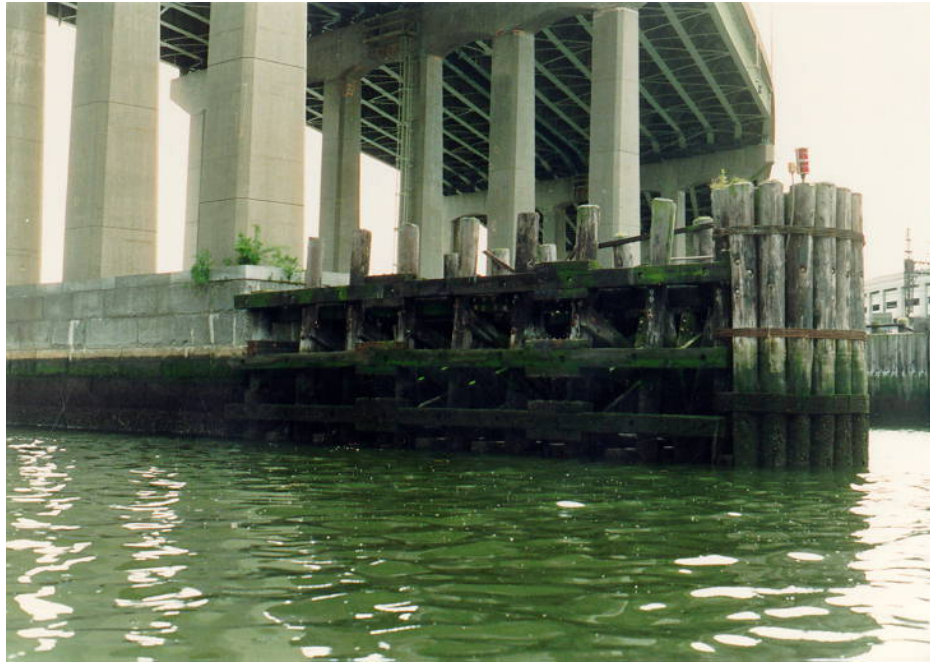
Figure 6.4.1a – Timber Fender System with Navigation Lights.
