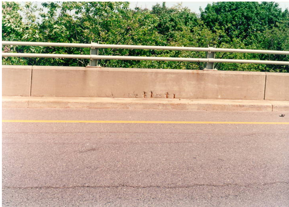
Figure 6.1.8a – Concrete Parapet with Older Style 2-Pipe Rail. Note Spalling with Exposed, Shallow Rebar.
