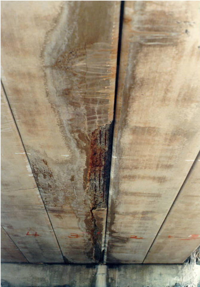
Figure 6.2.6a – Prestressed Concrete Deck Units with Severe Deterioration due to Leakage Between the Beams.
