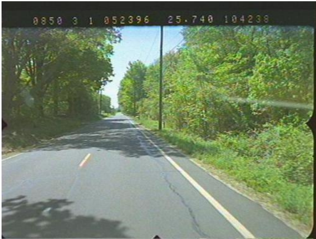
Photo 34 - 1996 DigitalHIWAY Image Note Location of Longitudinal Crack on Right
