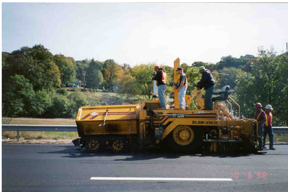
Photo A-4. Infrared Video Recorded From Top of Blaw-Knox PF-3200 Paver at Site 3.
