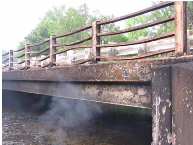
Figure 2. Photo. Bridge fascia immediately after fire.
