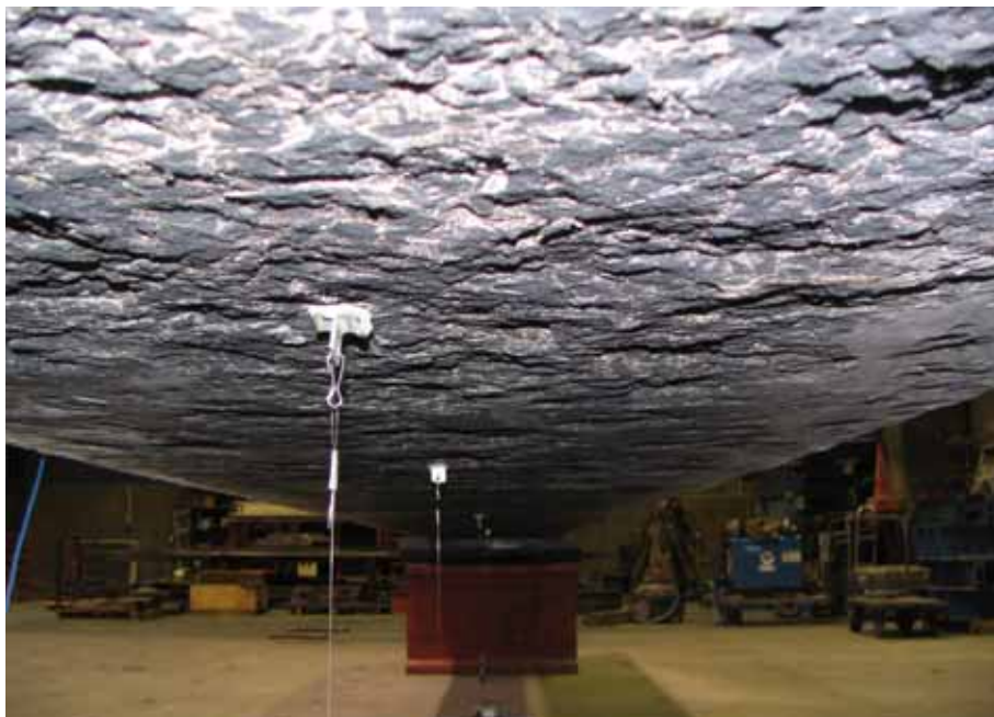
Figure 6. Photo. Bottom face of Beam 4.
