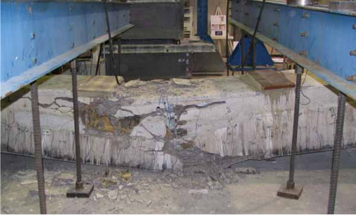
Figure 16. Photo. Failed Beam 4.
