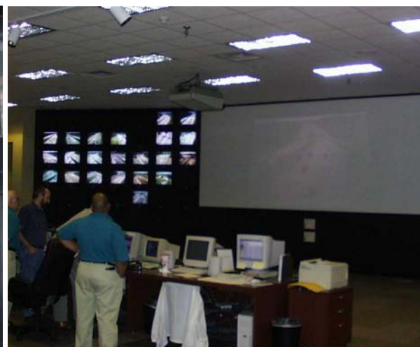
Figure 1b: Inside the Hampton Roads TMS
