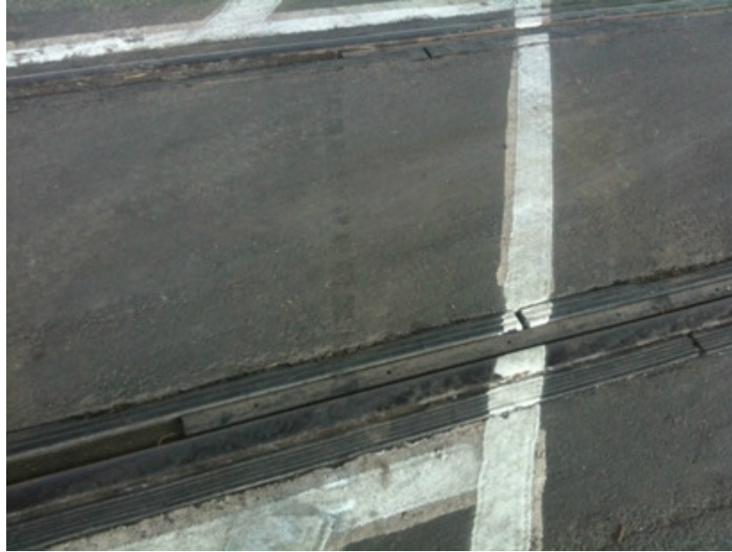
Rubber flange fillers were installed (Nov. 2011) in the rail flange ways in areas where cyclists could potentially pass over them.
