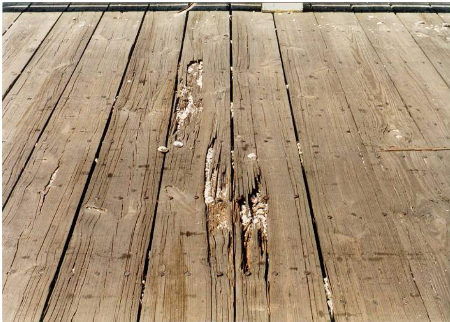
Figure 6.1.1a – Deterioration of Timber Plank Deck Surface
