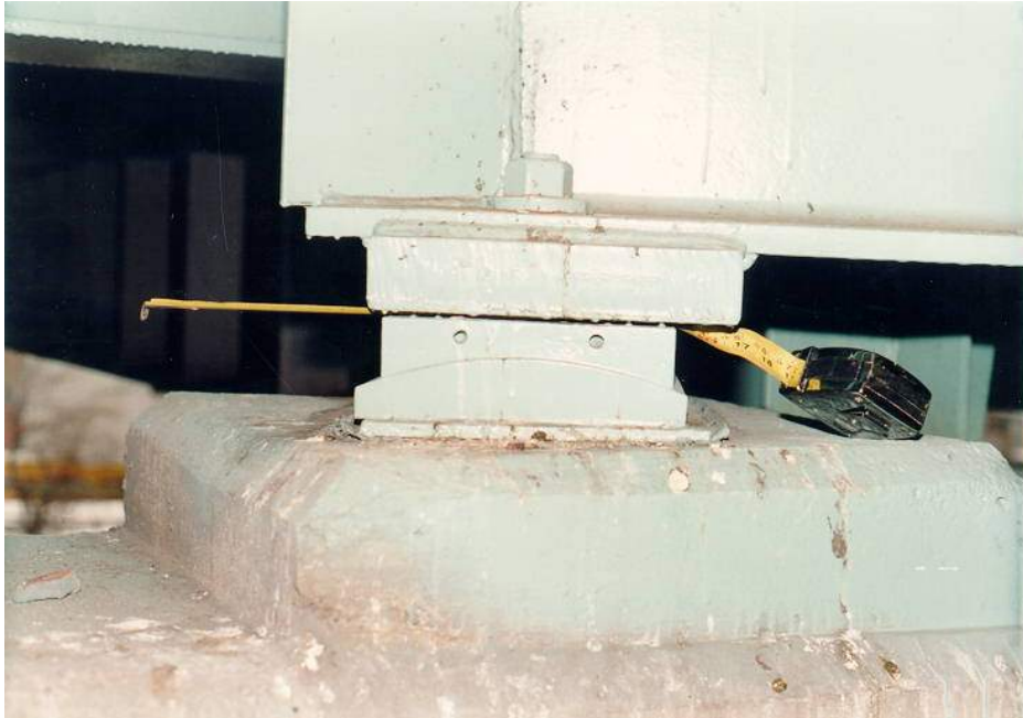
Figure 6.2.1j – Bronze Sliding Plate Bearing with a Gap Between the Sole Plate and the Sliding Plate.
