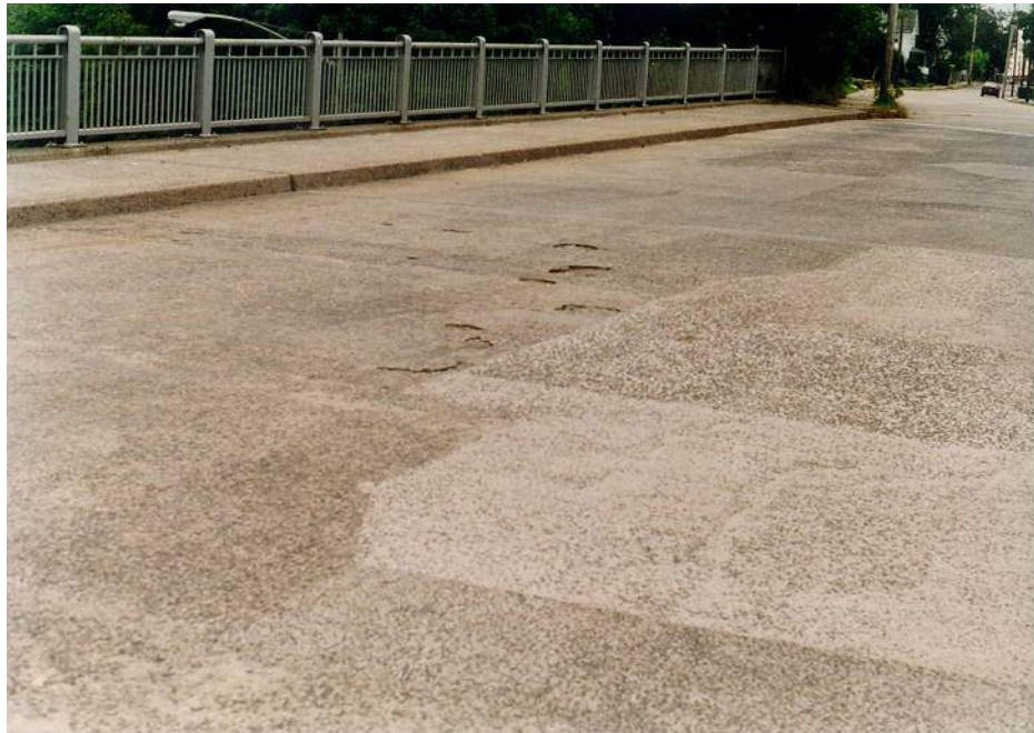
Figure 6.1.2b - Top of Bare Concrete Deck with Patched, Spalled and Hollow Areas.
