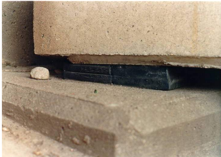
Figure 6.2.1m – Elastomeric Bearing. Note the Uneven Bearing Surfaces Causing Bulging and Cracking at the Rear of the Elastomeric Bearing Pad.
