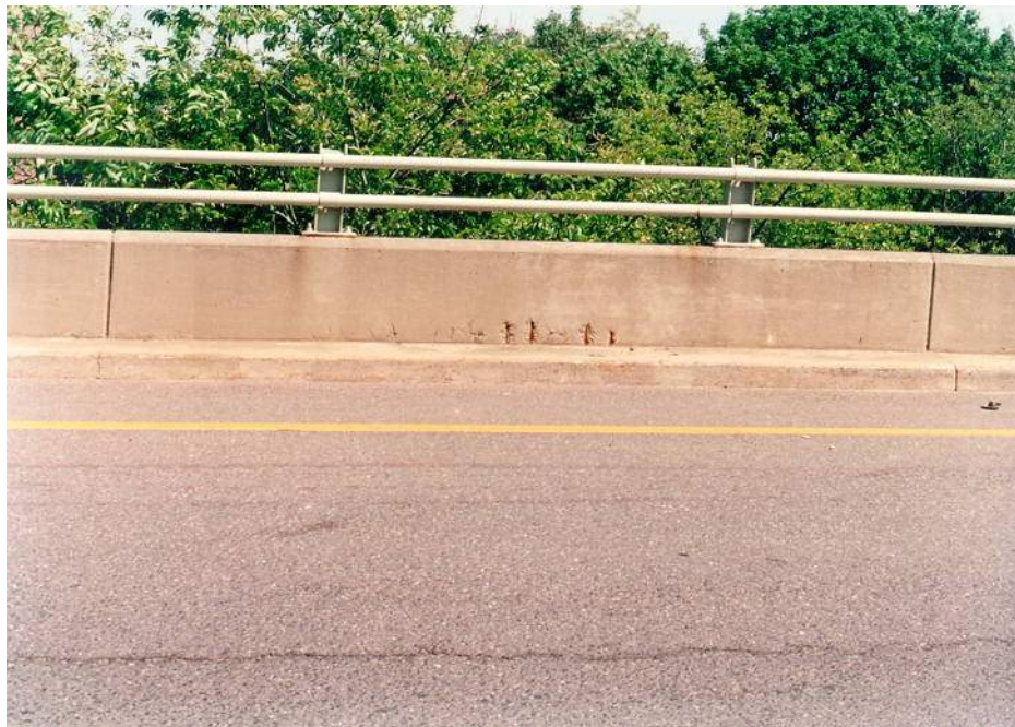
Figure 6.1.8a – Concrete Parapet with Older Style 2-Pipe Rail. Note Spalling with Exposed, Shallow Rebar.
