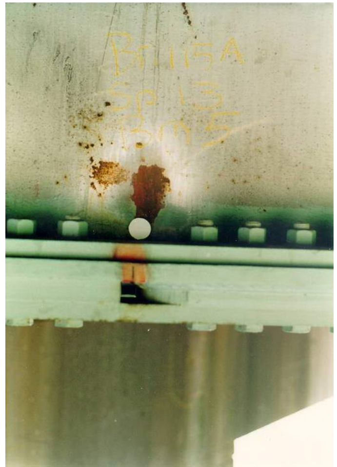
Figure 6.2.7.1c – Fatigue Crack Through the Bottom Flange of a Rolled Stringer at the End of a Partial Length Welded Cover Plate. A Stop Hole Has Been Drilled in the Web and Splice Plates Have Been Bolted to the Bottom Flange
