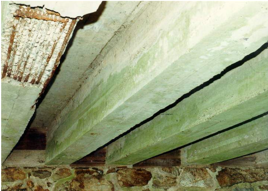
Figure 6.23a – Concrete T-Beams with Large Spalls Exposing the Bottom Layer of Reinforcing Steel.
