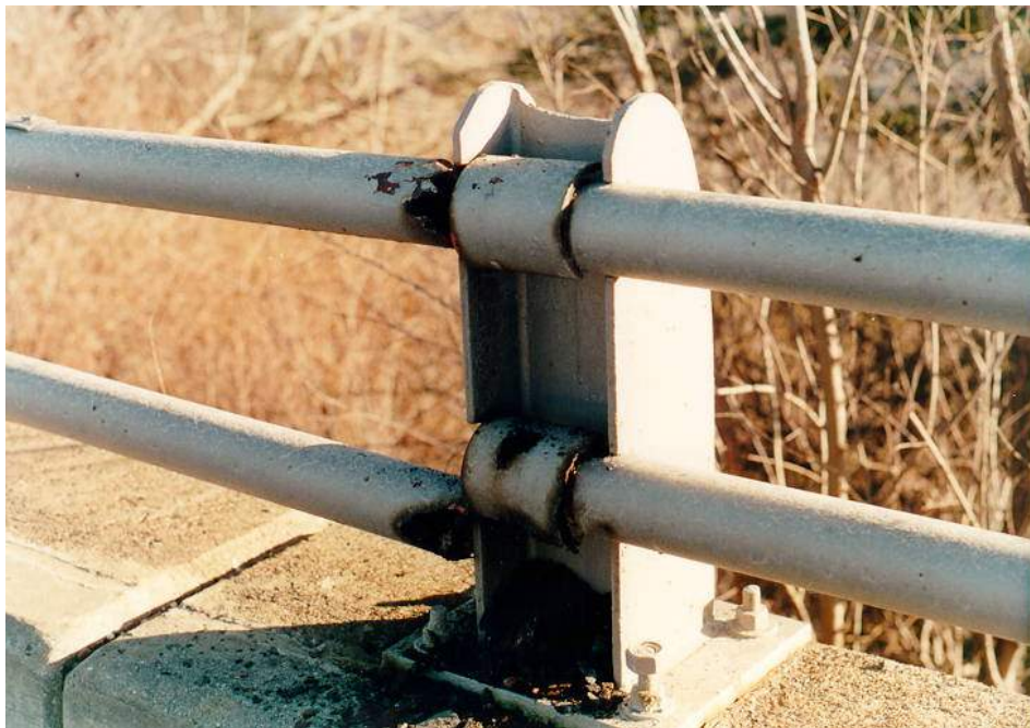
Figure 6.1.9a – Steel 2-Pipe Rail with Deterioration Frequently Found at Rail Posts.
