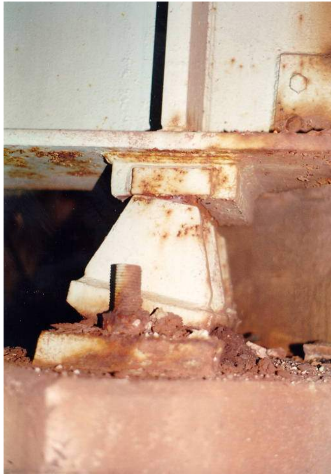
Figure 6.2.1i – Over Extended Rocker Bearing.
