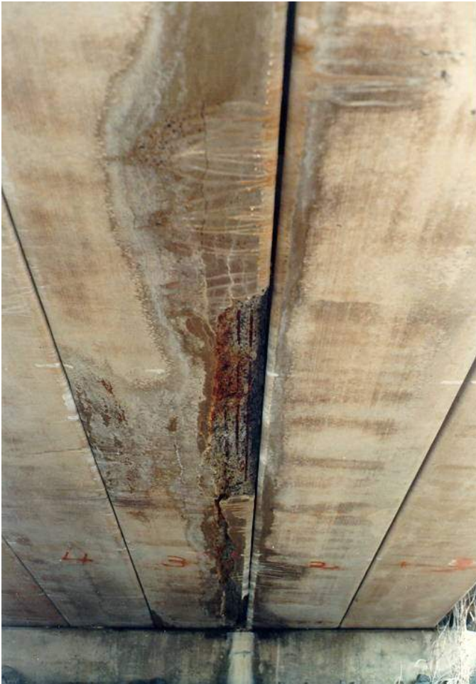
Figure 6.2.6a – Prestressed Concrete Deck Units with Severe Deterioration due to Leakage Between the Beams.
