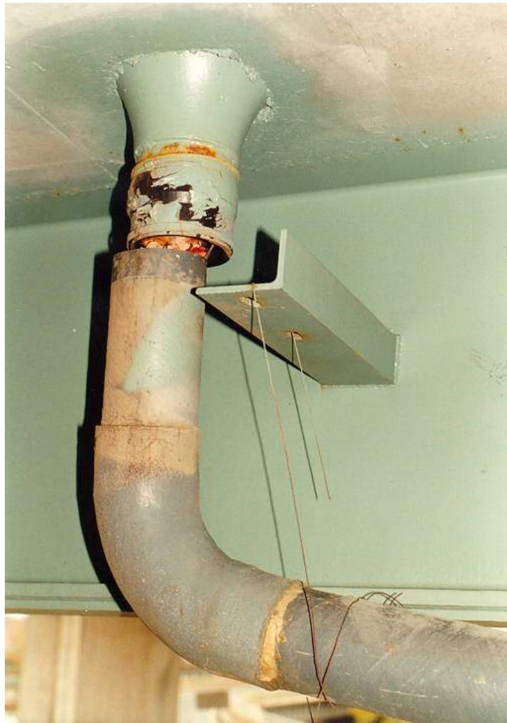
Figure 6.1.10a – Downspout Pipe Disconnected at Scupper Connection.
