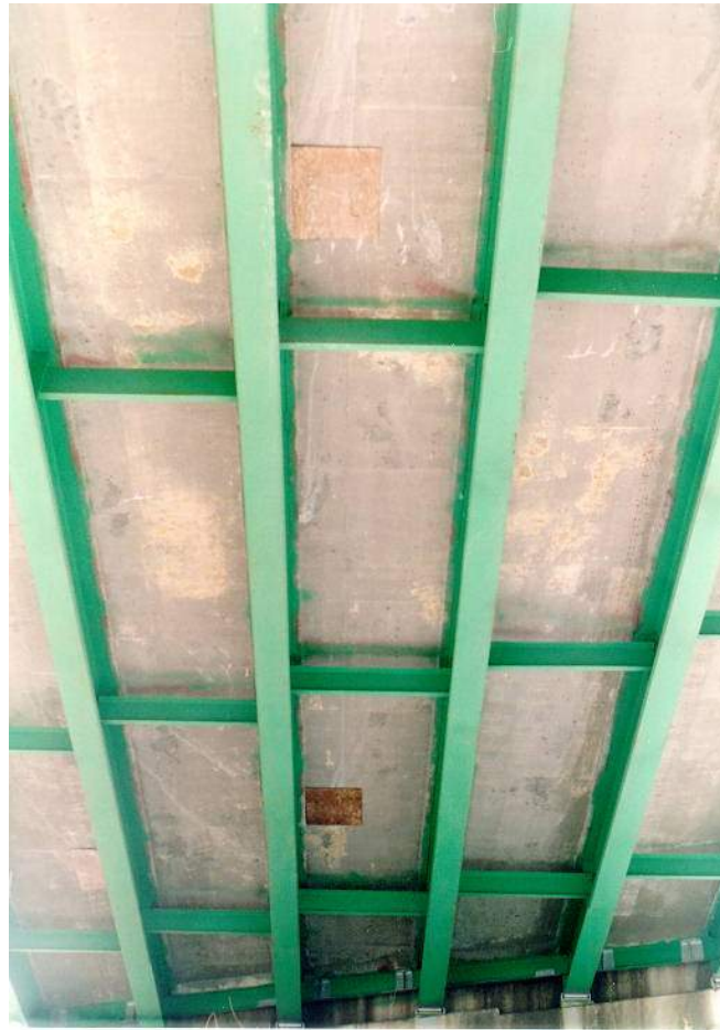
Figure 6.1.2c - Typical Underside of Concrete Deck. Note Cracking with Efflorescence and Formwork Remaining from Full Depth Patching.
